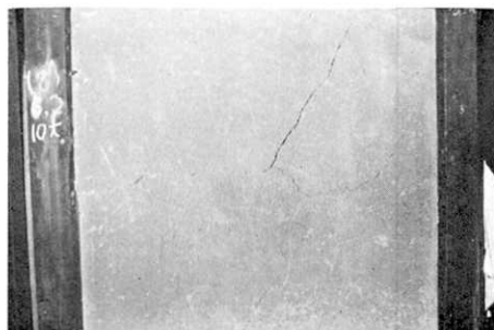
Fig. 19. Cracks in mud wall
