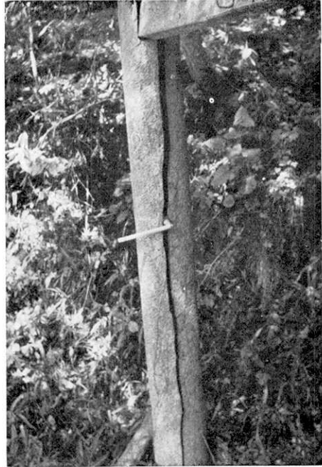
(b) Vertically cracked stone column of Torii at Taki (width: about 2 cm).
