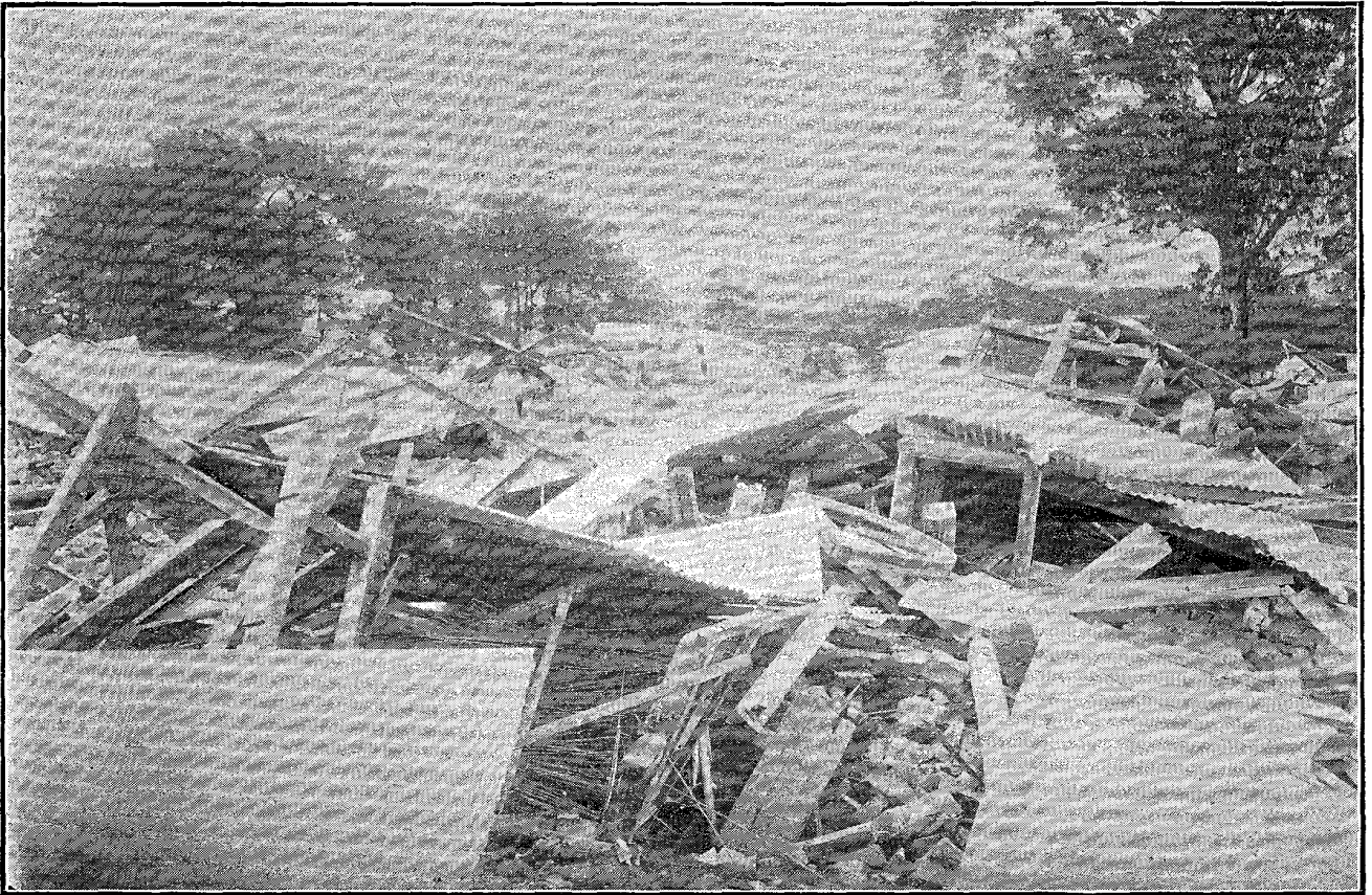
Fig. 27. The Gazette, Office, Shillong. (After the earthquake.)
