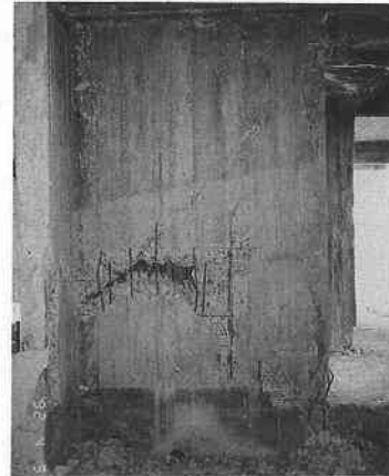
Photo 12 Shear failure in the central core wall
