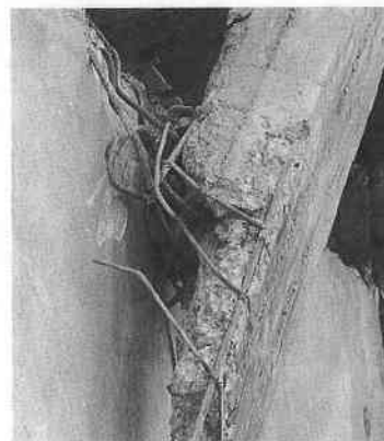
Photo 4 Close-up view of column with pullout failure due to inadequate anchorage of column reinforcement to beam
