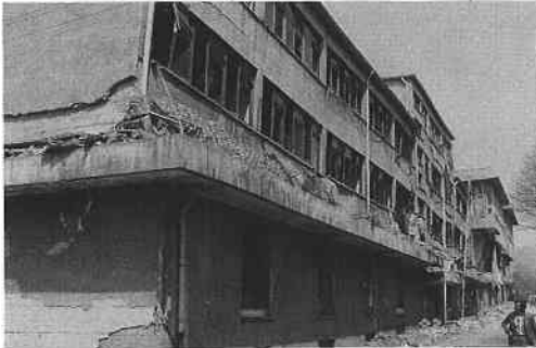
Photo 6 Communication Building collapsed in the second story [Karaagac District]
