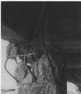
Photo 8 Buckling of longitudinal bars due to absence of lateral reinforcement in beam-column joint
