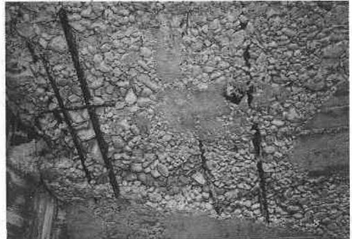
Photo 10 Honeycombs exposing embedded reinforcement
