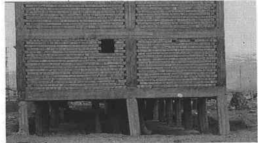
Photo 9 Soft story failure
