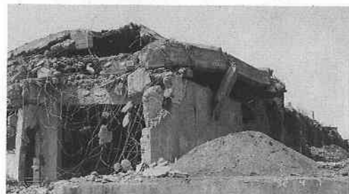
Photo 3 Residential building collapsed in upper stories [Kizilay District]
