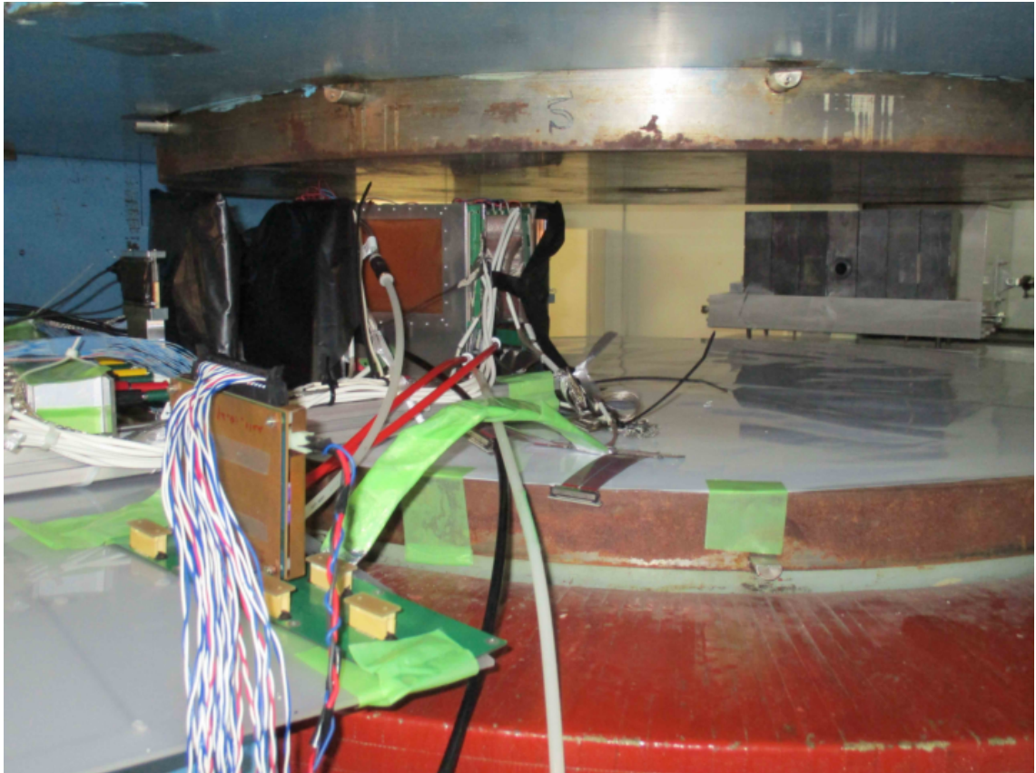
Figure 3.6: Detectors installed in a RTAGX dipole magnet. The jig is placed according to a life-size printed drawing fixed on a pole.
