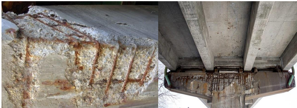
Figure 1.1 spalling of concrete in corroded RC structure [9]
