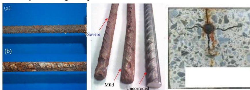
Figure 1.2 Different level of corroded reinforcing bar and corrosion crack from expansion of corroded bar [10,11]
