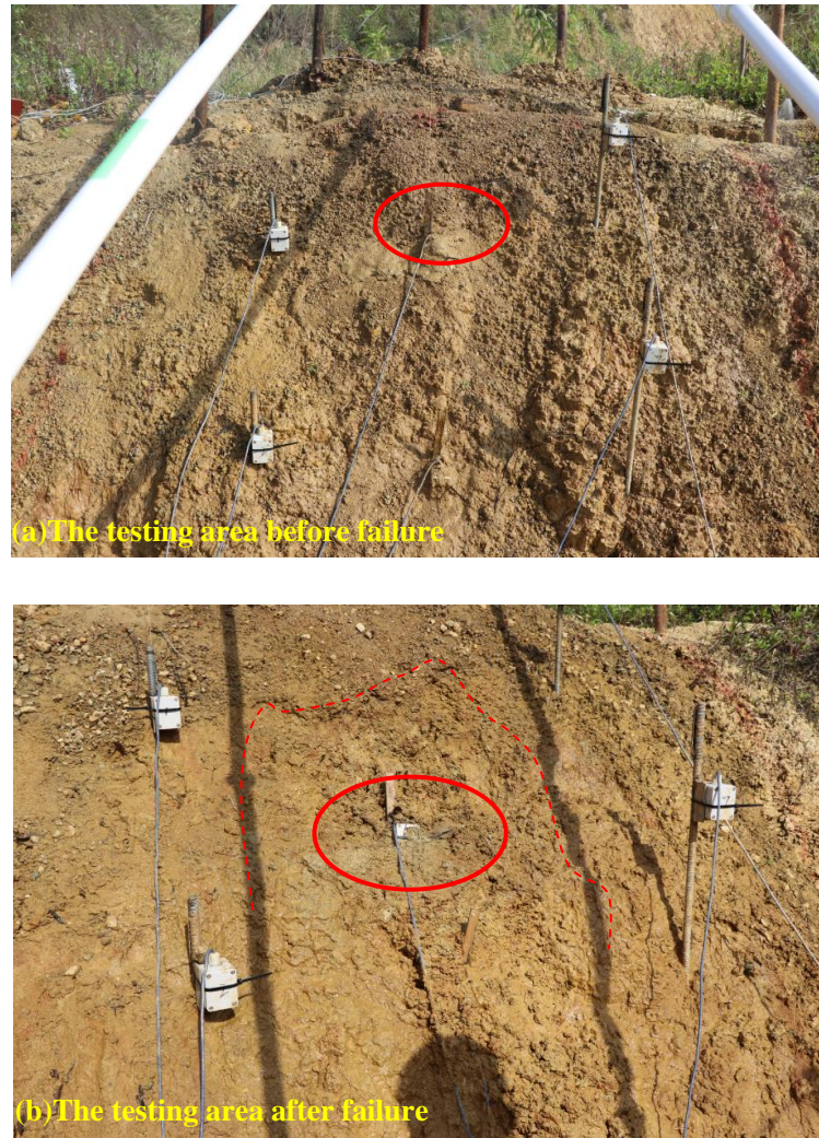
Fig. 5-44 Images of the testing area before and after the slope failure
