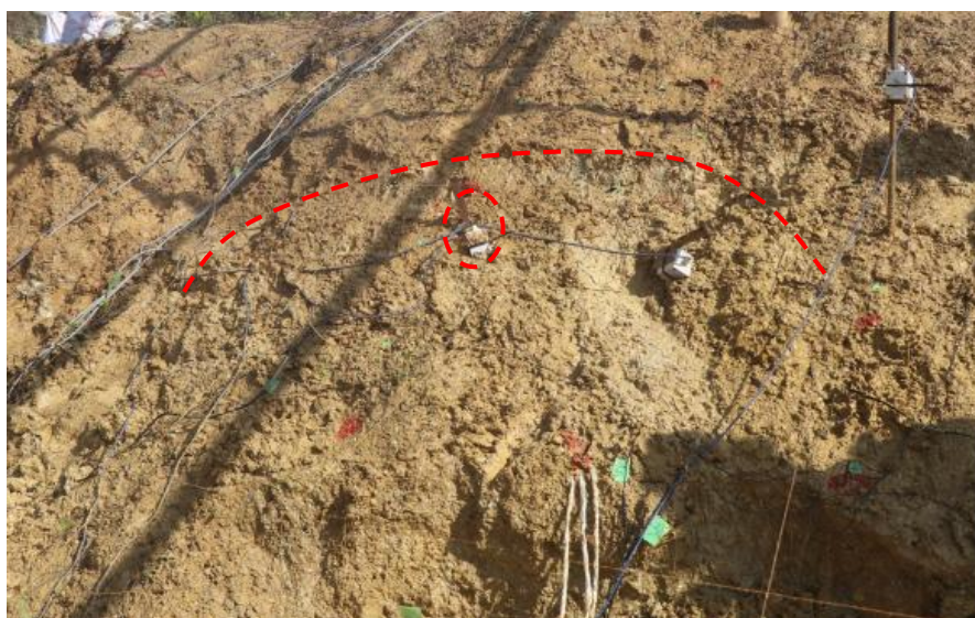
(b) The image for the testing site after slope failure
