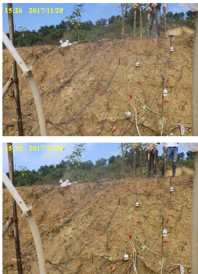
Fig. 5-48 Erossion occurred in lower part and caused the tilt sensors failed
