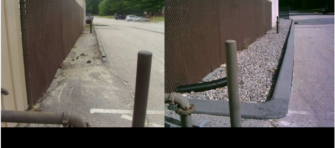
Figure 5-6. Infiltration BMP to capture and infiltration of runoff from parking lots (Picture provided by Mr. Don Morris, USAF and picture taken during Dec. 2013 filed visit.)
