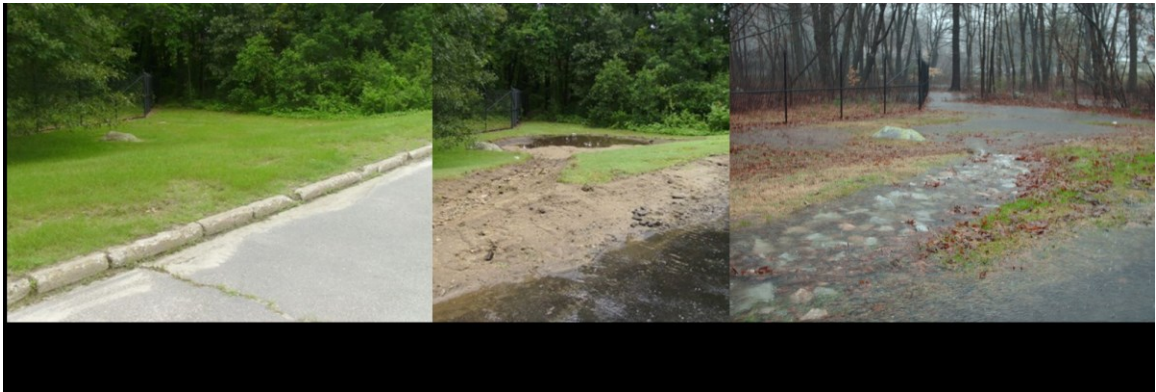
Figure 5-7. Infiltration BMP to capture and infiltration of runoff from parking lots (Pictures provided by Mr. Don Morris, USAF)
