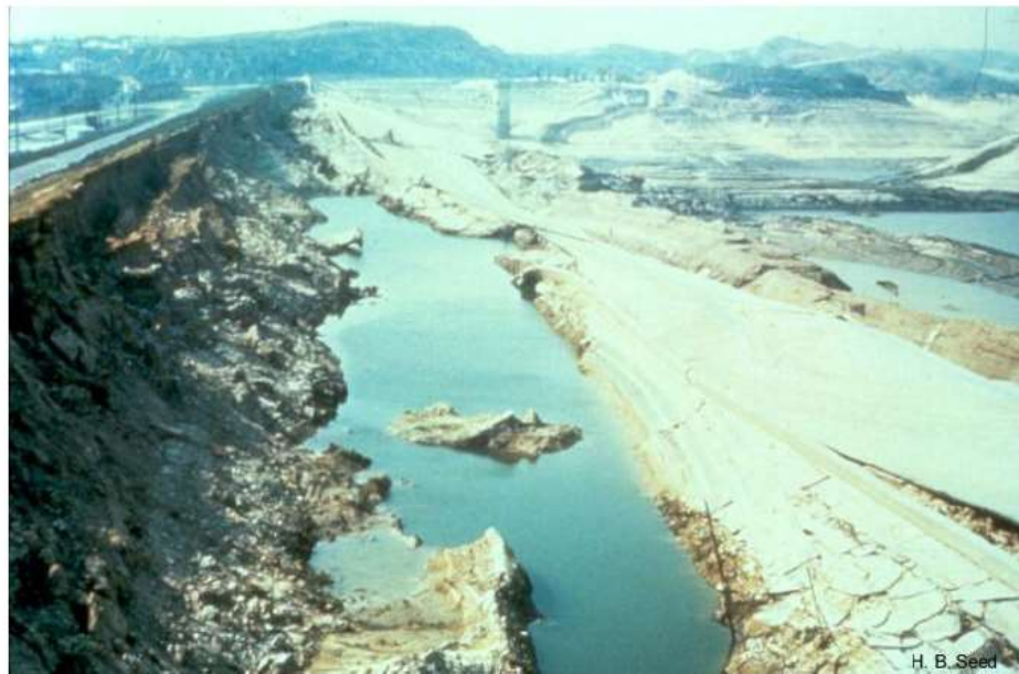
Figure 1.2: Upstream face of the dam after drawing down the reservoir (Pic courtesy to H.B Seed)
