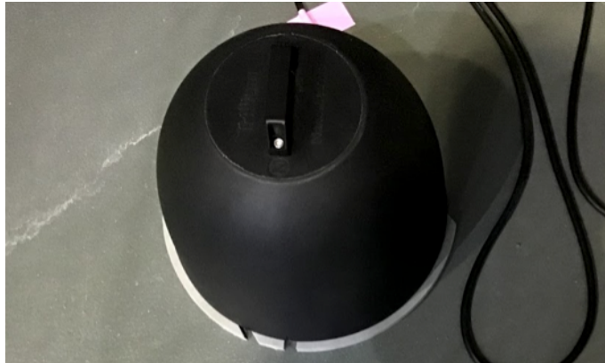
Figure 2.10: Trillium 120-QA installed on the second floor at X-end area, which is covered by black thermal insulation cover
