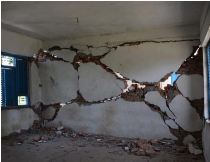
Cracks on the infill walls
