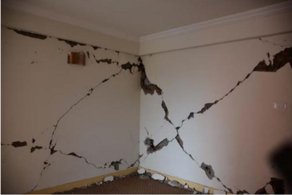
Cracks on the infill walls
