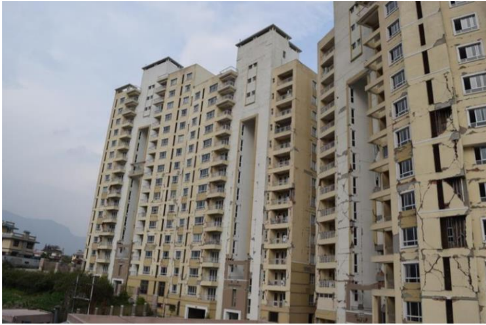
Figure 1.10 (b) Structural and non-structural damage in the Park View Horizon apartment building at Dhapasi, northern part of the Kathmandu valley (Hashash et al. , 2015).
