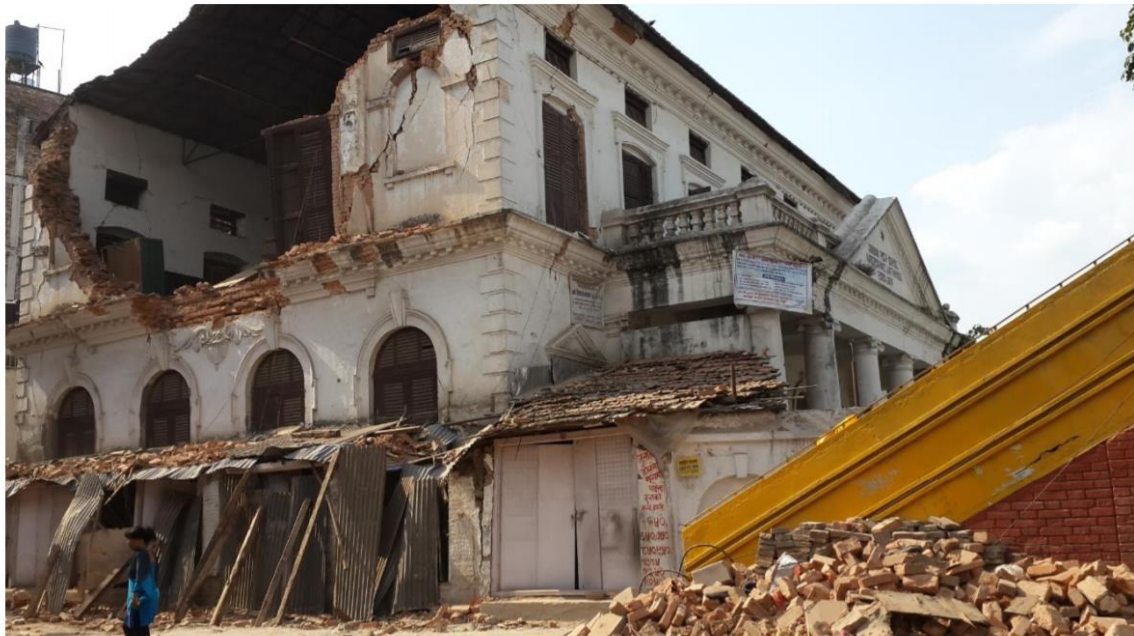
Damaged School Building (Durbar High School) in the central part of the Kathmandu valley at a distance of 527 m south-west of the Kantipath (NQ.KATNP) strong motion station.
