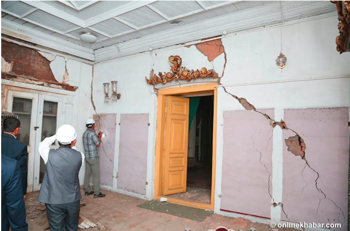
Damaged observed in Hanuman dhoka durbar in Kathmandu Durbar square (online khabar.com)
