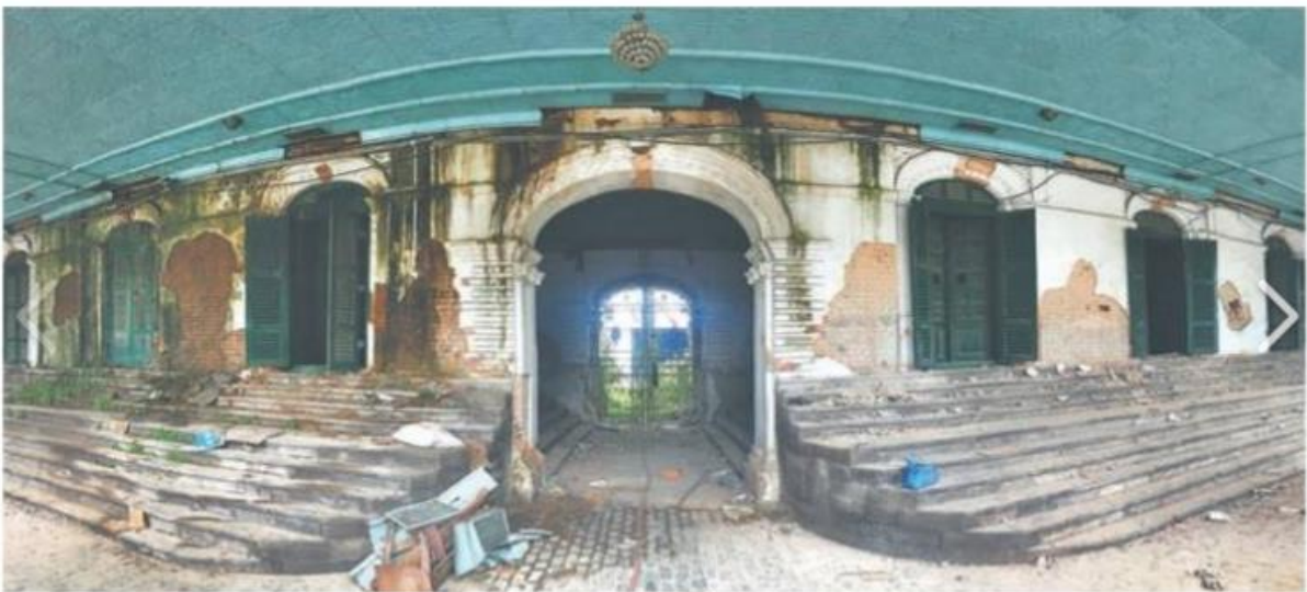
Damaged buildings in the periphery of Singhadurbar
