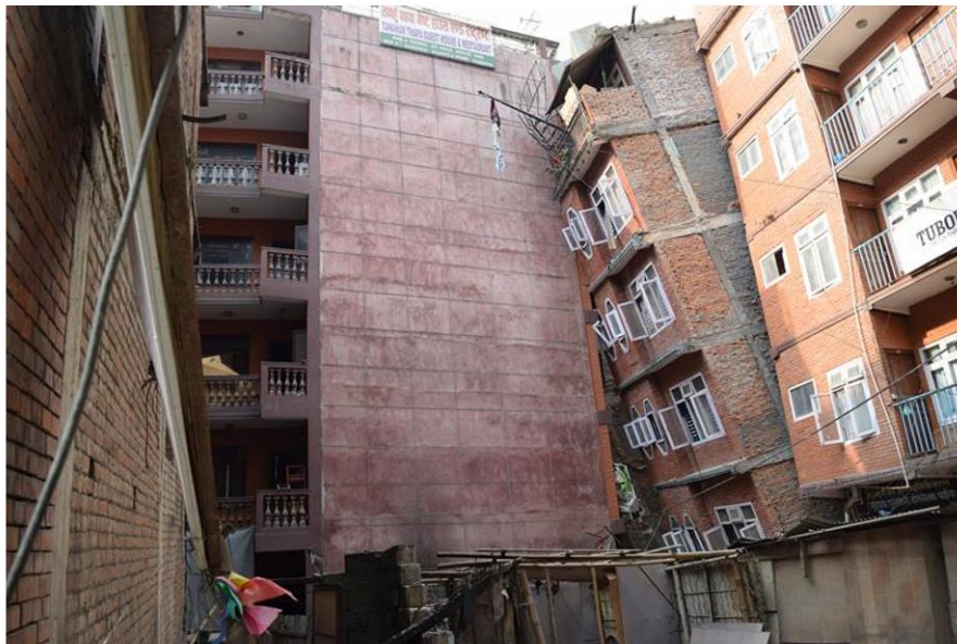
Figure 1.10 (c) Soft-story collapse of a 6-story building in Balaju near the Gongabu bus terminal (new bus park) one of the heavily damaged areas in the Kathmandu valley killed over 20 people in the neighbourhood (Hashash et al. , 2015).
