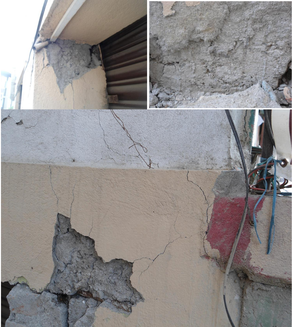
Damage in the RC buildings
