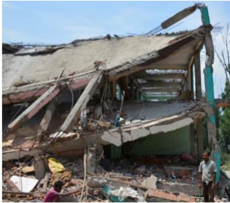
Pan-cake Collapse of the residential building in the Kathmandu valley
