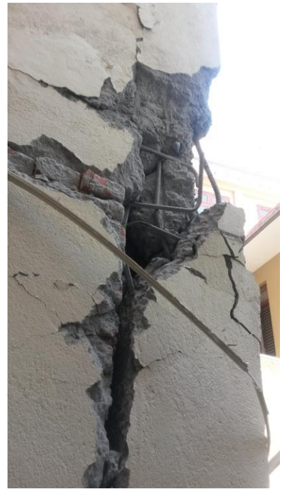
Damage in the various RC and load bearing buildings
