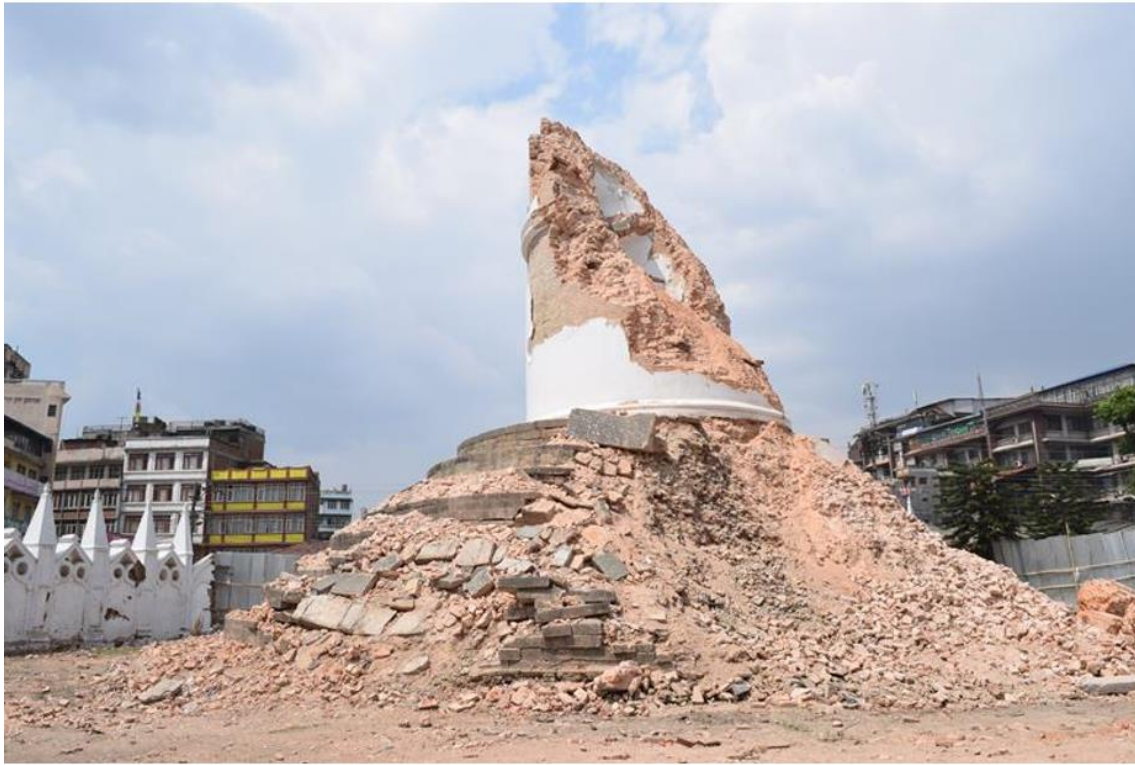
Figure 1.10 (a) Residuals of the sixty-meter-high 9-story historical Bhimsen tower (Dharahara) in the central part of the Kathmandu valley after the Gorkha earthquake (Hashash et al. , 2015).
