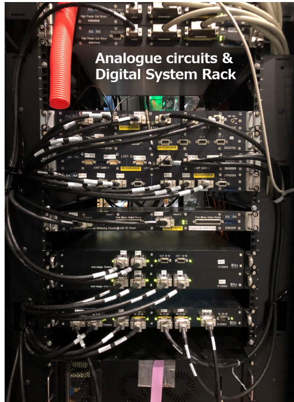
Figure 5.36: An example of in-air cabling around the rack that houses the analog circuits to drive the sensors and actuators.
