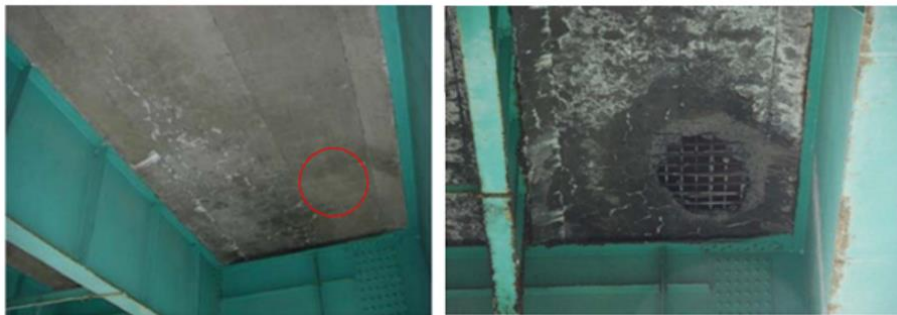
Figure 7-33 Punching shear failure happened within 5 years
