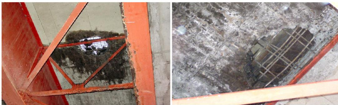
Figure 1-3 punching shear failure of RC slab
