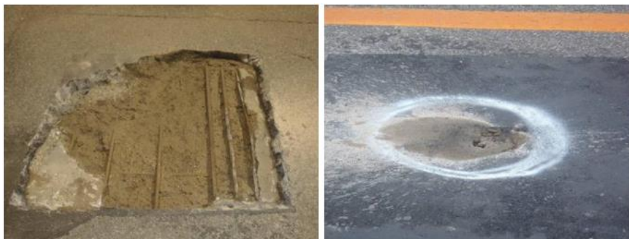
Figure 1-2 damage cases of steel bridge RC deck
