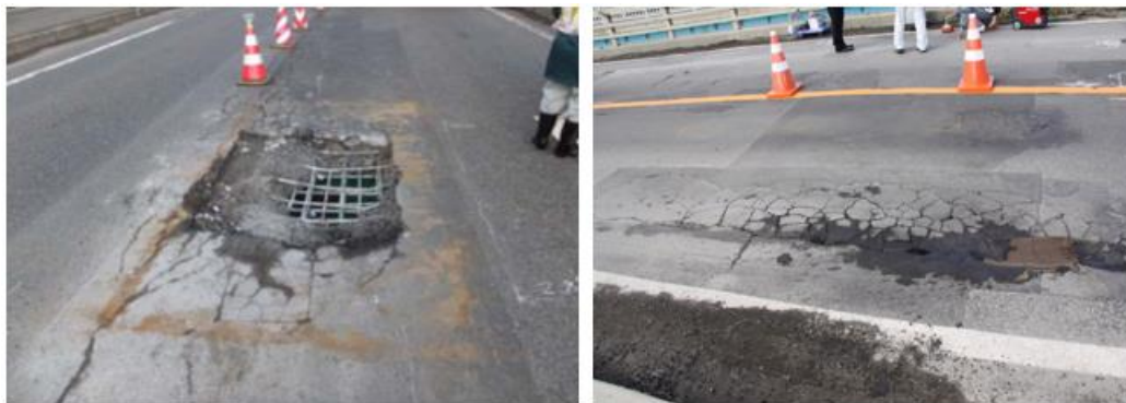
Figure 3-2 deterioration example in East Japan
