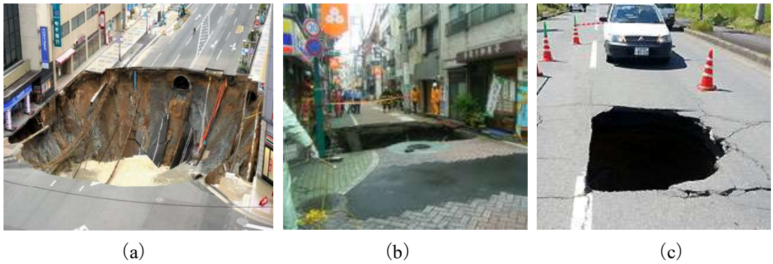
Fig. 1.5 Road collapses (a) Fukuoka prefecture (b) Tokyo prefecture (c) Kyoto prefecture 9)-11)
