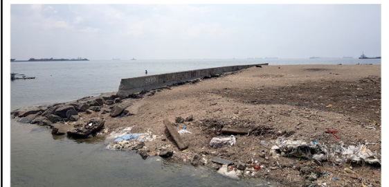
Dilapidated seawall along Points C2 to C5.
