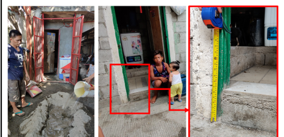
Residents pouring concrete in order to elevate the floors of their houses. Measured elevated floor is Point E5.
