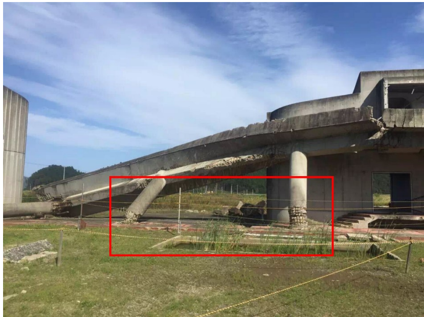
Fig. 1.1 Photograph taken at Ohgawa Elementary School after the 3.11 Tohoku tsunami, Miyagi prefecture, Japan
