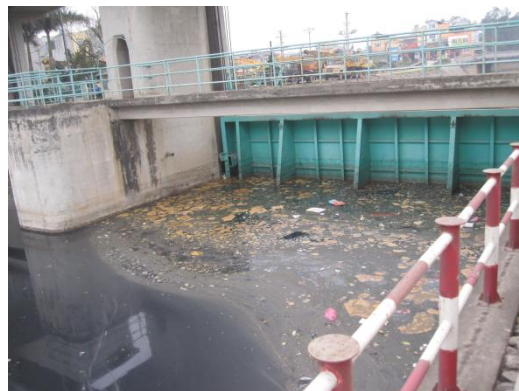
Figure 11. Thanh Liet water gate
