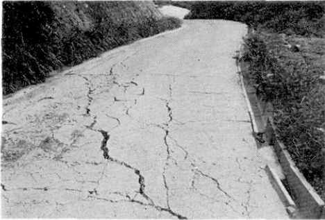
Fig. 35. Damaged pavement and ditches on the fault line at Loc. N-6.
