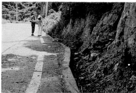
Fig. 20. Fault outcrop and displaced road at Loc. 13.
