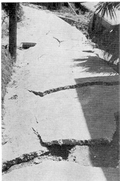
Fig. 43. Cracks in the road at loc. G-6.
