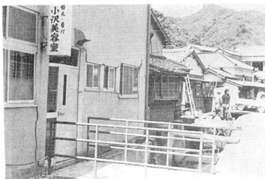
Fig. 34. Destruction of a mortar wall at loc. S-10.
