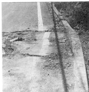
Fig. 53. The right lateral displacement on the road at loc. G-10.
