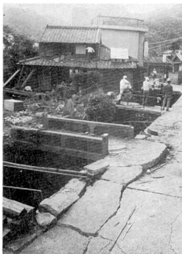
Fig. 31. Cracks in the road at loc. G-2 and the damage to houses.
