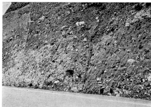
Fig. 87. Small faults and a small crack in the road at loc. R-15, showing lateral displacements of small amounts.
