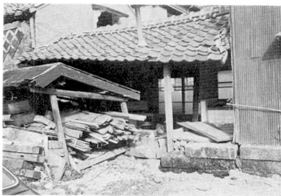
Fig. 29. Lateral displacement of the foundation blocks at loc. S-6.
