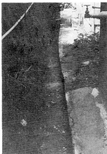
Fig. 93. Destruction and distortion of a trench at loc. S-29 (already repaired).
