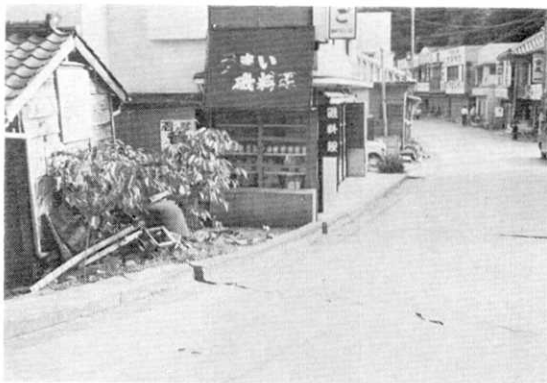
Fig. 28. Cracks in the road at loc. G-1.
