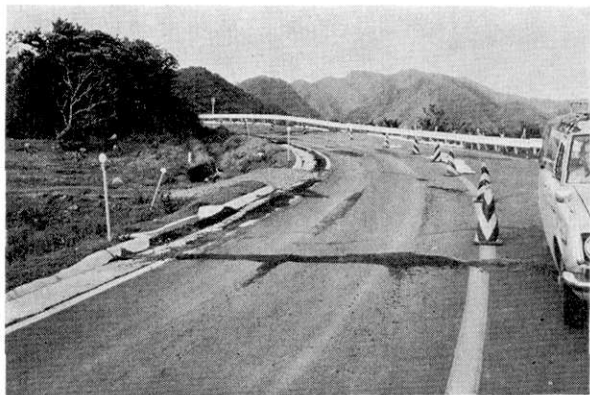
Fig. 89. Cracks in the road at loc. G-33.
