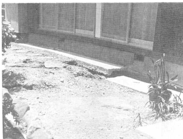
Fig. 39. Fissures in the ground at loc. S-15.
