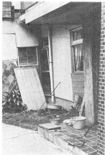
Fig. 27. Destruction of a mortar wall and cracks in the ground at loc. S-2.
