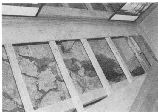
Fig. 41. Fissures in the ground at loc. S-15.
