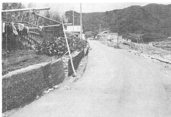
Fig. 74. Cracks in the road and the destruction of a concrete fence at loc. G-26.
