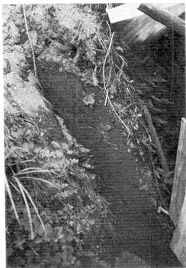
Fig. 48. Earthquake fault at loc. R-4.
