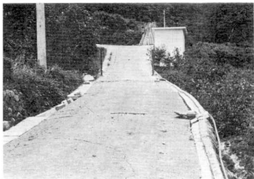
Fig 56. Cracks in the road at loc. G-12.
