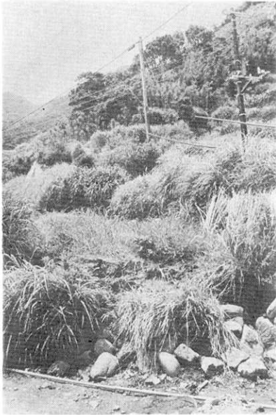
Fig. 79. Destruction a of masonry retaining wall and slides, at loc. G-29.
