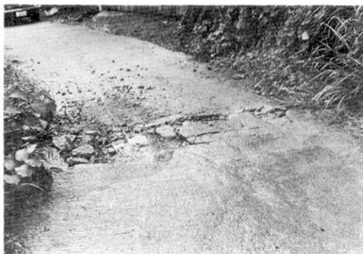
Fig. 86. Cracks in the road at loc. G-31.
