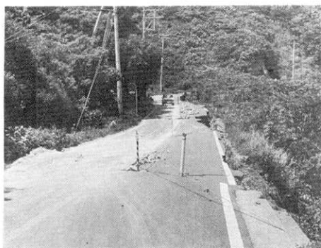
Fig. 6. Destruction of a road at Oku-Irozaki.
