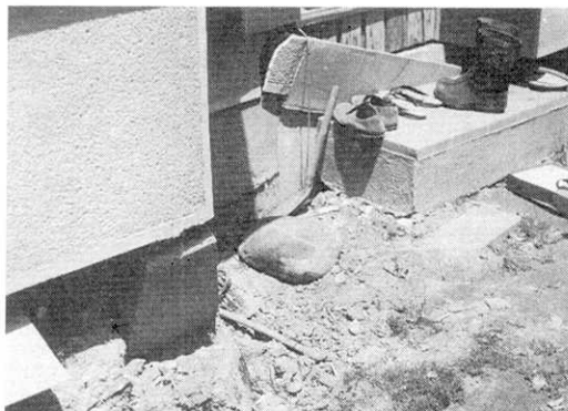
Fig. 51. Destruction of the concrete foundation at loc. S-19.
