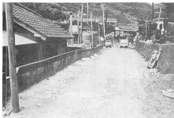
Fig. 76. Cracks in the road and the destruction of a concrete fence at loc. G-27, showing right lateral displacement.
