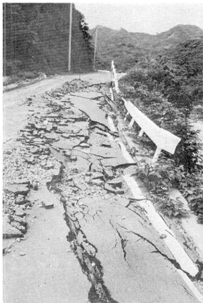
Fig. 64. Destruction of the road at loc. G-20.
