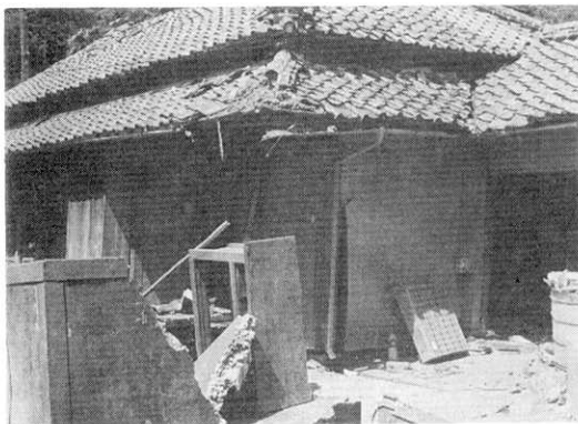
Fig. 32. Destruction of a house and the concrete fence at loc. S-8.
