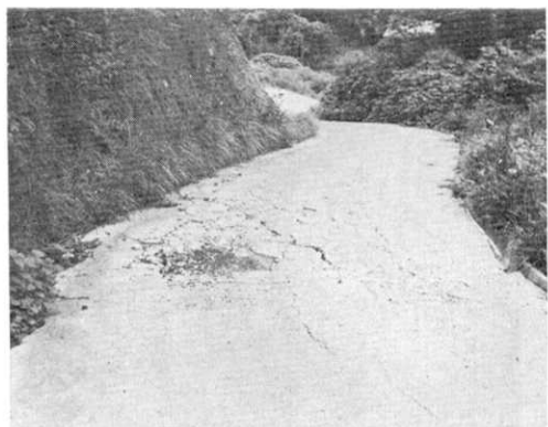
Fig. 58. Cracks in the road at loc. G-14.
