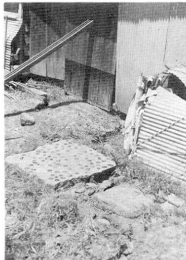
Fig. 47. Fissures in the ground and damage of a house at loc. S-18.
