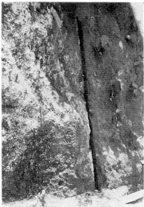
Fig. 55. Earthquake fault at loc. R-6.
