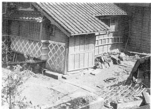
Fig. 4. Sliding of a house from the foundation blocks at Iruma.
