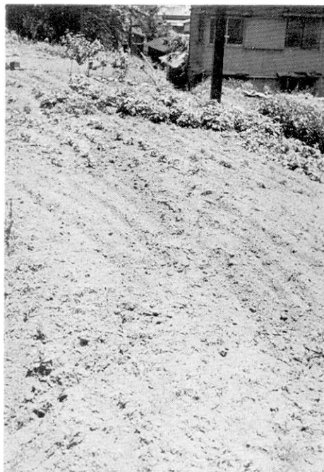
Fig. 45. Fissures in the ground at loc. G-7.
