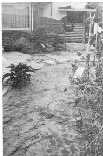
Fig. 37. Fissures in the ground at loc. G-4.
