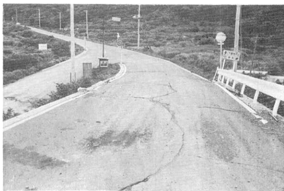
Fig. 66. Cracks in the road at loc. G-20.
