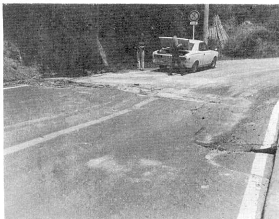
Fig. 52. Cracks in the road at loc. G-10.
