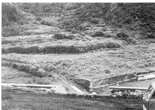
Fig. 71. Destruction of a concrete embankment at loc. S-24.
