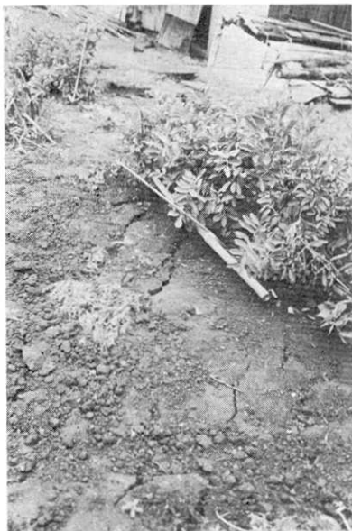
Fig. 46. Fissures in the ground at loc. G-8.
