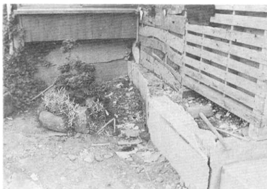
Fig. 38. Destruction and lateral displacement of a concrete foundation and mortar wall at loc. S-13.
