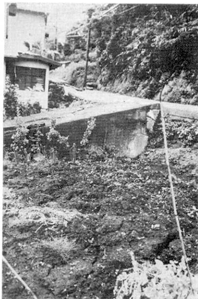
Fig. 44. Fissures in the ground at loc. G-5.
