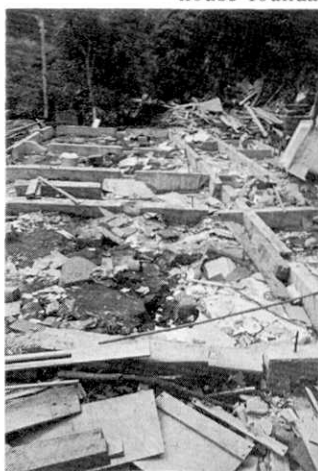
Fig. 29. Fault crack which destroyed a house foundation.
