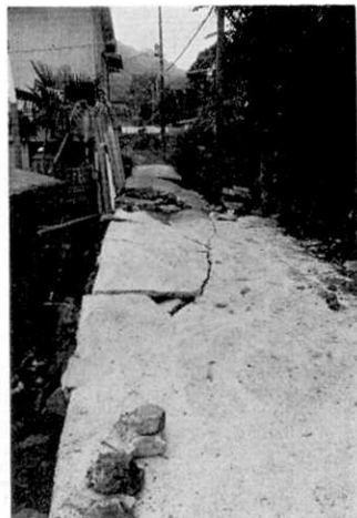
Fig. 33. Concrete pavement destroyed by fault.
