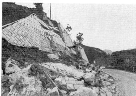
Fig. 9. Damage to a slope protection.
