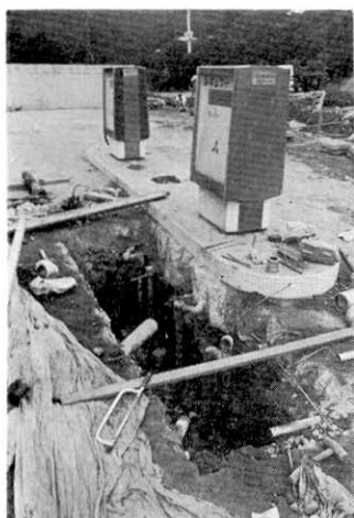
Fig. 27. Damage to an underground pipe connection at a gas station.
