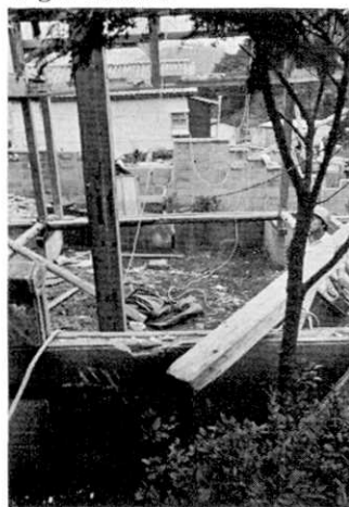
Fig. 31. Fault crack which destroyed a block fence and house foundation.
