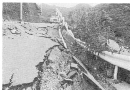
Fig. 5. Settlement of a road surface.
