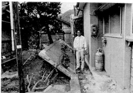
Fig. 57. Overturning of a concrete fence at Iruma Village.
