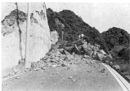
Fig. 10. Fallen stones on road.
