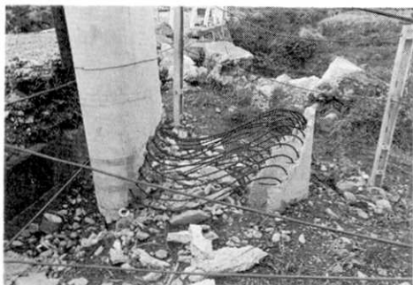
Fig. 26. Damage to an electric pole.
