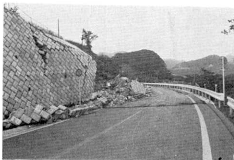
Fig. 8. Damage to a slope protection.
