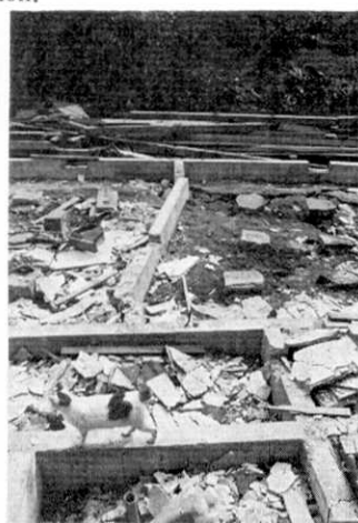
Fig. 30. Fault crack which destroyed a house foundation.
