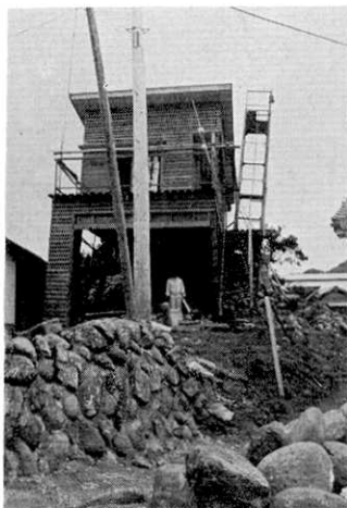
Fig. 53. Inclination of a house caused by the destruction of stone pitching.
