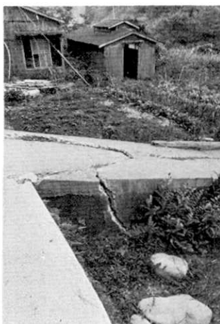
Fig. 32. Crack in a field surface and in concrete produced by a fault.
