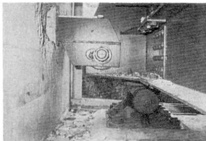
Fig. 15. Damage to a protection device which prevents a girder from falling.
