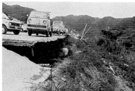
Fig. 54. Slide of the supporting soil of a parking lot.
