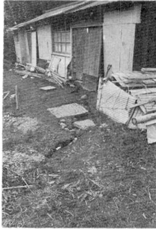
Fig. 36. Fault passage through a wooden house.
