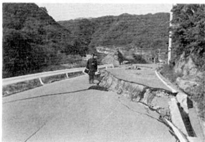
Fig. 3. Crack and sliding of embankment part.
