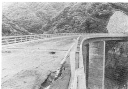
Fig. 11. Settlement of soil by 30 cm behind bridge abutment.
