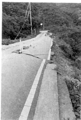
Fig. 2. Crack on road surface and settlement of embankment.
