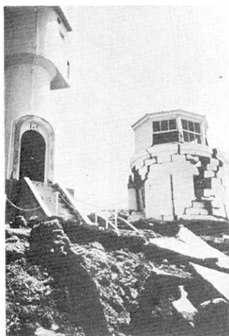
Fig. 5. Collapsed block wall of the observatory at Irozaki.
