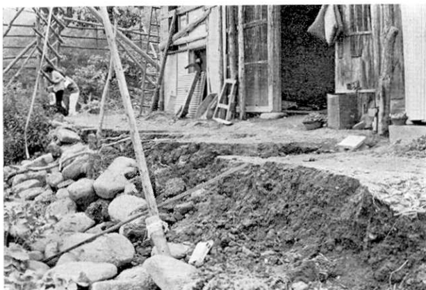
Fig. 12. Failure of the fill-up foundation of a house, at Iwaigawa.
