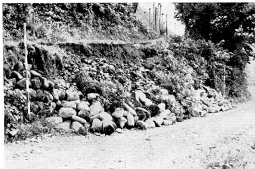
Fig. 7. Failure of the masonry retaining wall at Hirukawa.
