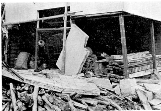
Fig. 13. Failure of the barn wall made of concrete-block at Iwaigawa.
