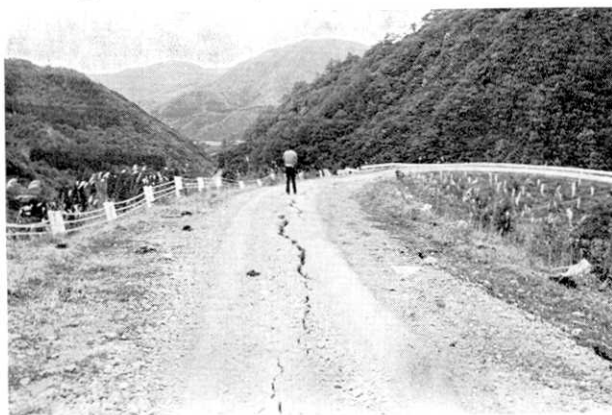
Fig. 19. Occurrence of cracks on the road to the east of Iwaigawa.
