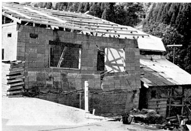
Fig. 22. Failure of the wall made of concrete-block at Yukawa, Yuta-machi. A crack transversing on the asphalt road was due to the subsidence of roadbed.
