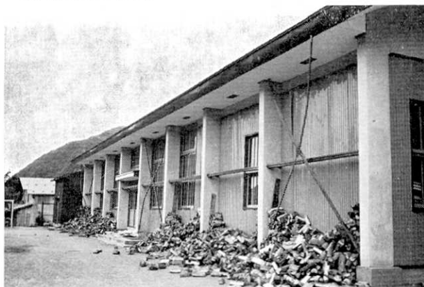
Fig. 18. Failure of the iron diagonal beams at Iwaigawa Elementary School.
