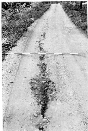
Fig. 6. Occurrence of a crack due to the slide of the roadbed at Hirukawa, Higashinaruse-mura.
