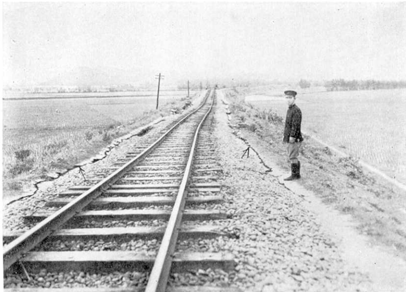
第 62 圖 竹南淡文湖間鐵道被害. Fig. 62. Damages of railway near Tikunan.
