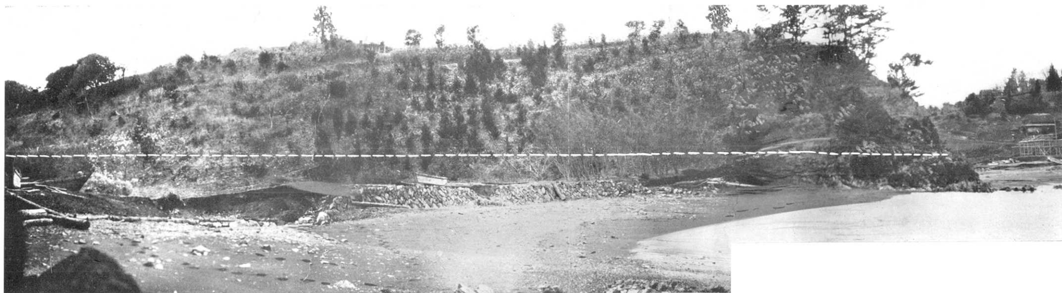
第 353 圖 唐桑村石濱區砂子濱附近の海岸. 津浪は小山の下部を洗ひ海岸護岸工事を大破してゐる. 津浪痕跡は圖中白線で示めす所に見られ, 浪高は 8.1 米. (4 月 20 日西村, 高山撮影) Fig. 353. Beach near Sunakohama, Karakuwa village. White line shows heights at which traces were left by tsunami. Sea wall destroyed. Wave height 8.1 meters. (Photo by G. Nishimura and T. Takayama, April 20.)
