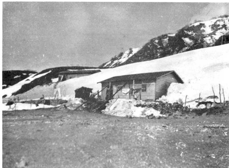
第 218 圖 庶野の家屋. 前面は大半修理してある. (4 月 6 日那須撮影) Fig. 218. House at Syoya. Front side of this house was ripped off by tsunami waves. (Photo by N. Nasu, April 6.)
