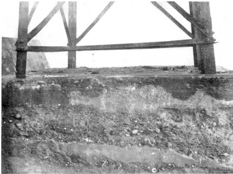
第 225 圖 幌泉港入口燈臺の脚部に附着せる海草其他の流漂物 (4 月 4 日那須撮影) Fig. 225. Seeweeds and other debris attached to the foot of the light-tower at the entrance to the port of Horoidumi. (Photo by N. Nasu, April 4.)
