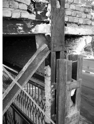
Photo 8. Fracture of welded joint of a steel brace.
