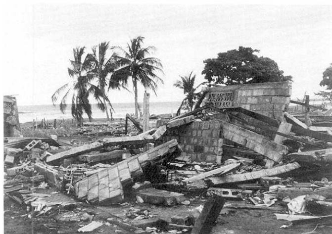
Photo. 6. Broken down block fence at El Transito.
