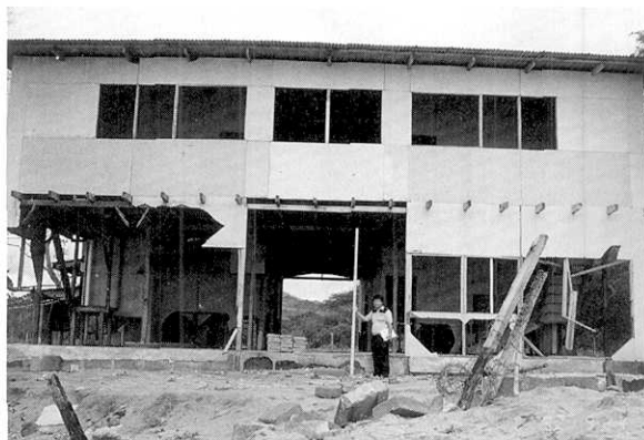
Photo. 9. Seriously damaged house on the coast of Marsella Bay (D in Fig. 33). Sea water passed through the first floor of the house.
