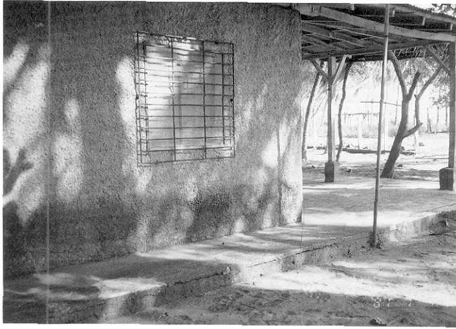
Photo. 1. Trace of tsunami on a wall at Jiquilillo.
