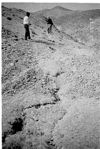
Photo 27. Fissures on the upper slope of a mountain north of Pakdeh (Site No. 2 in Fig. 7). Looking north. The fissures are aligned in several strips trending N-S, extended further across the northern valley.
