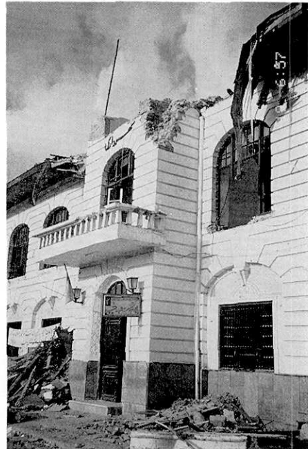
Photo 14. City Hall of Rasht. Two-storied wooden frame masonry structure looking southwest. The heavy cap made of brick at the entrance hall fell down on the pavement in front.
