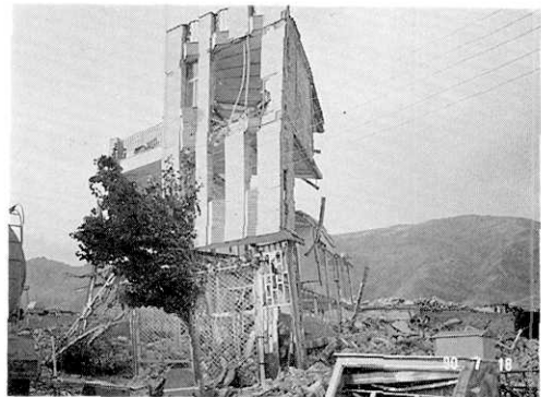
Photo 17. Damage to a two-storied steel frame building in Manjil. Roofs, floors and bearing walls collapsed.
