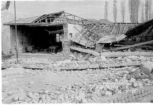
Photo 18. Destroyed elementary school building in Pakdeh (Site No. 3 in Fig. 7). The brick walls collapsed. No bracing in the wooden structure under the roof.
