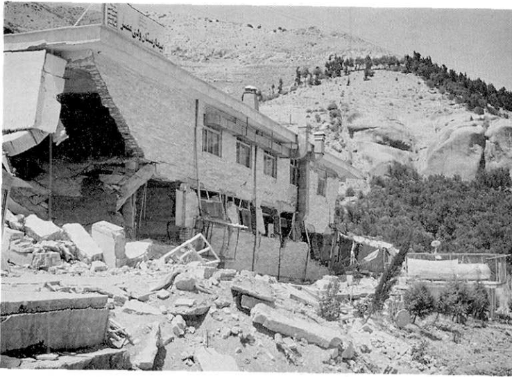
Photo 15. Damage to a two-storied building of the Vali-e-Asr Hospital in the suburbs of the City of Rudbar (Site No. 5 in Fig. 6). Looking northwest.
