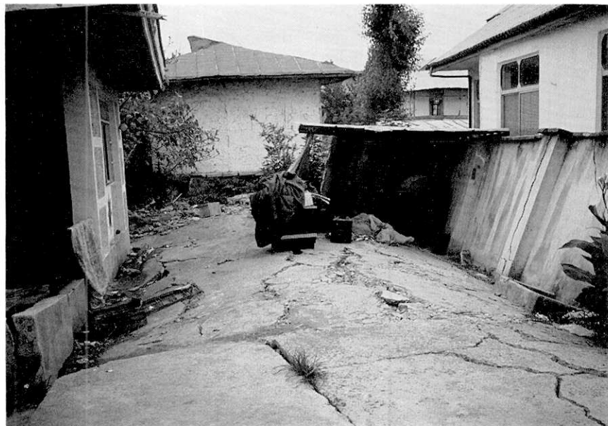
Photo 33. Ground uplift due to liquefaction in Astaneh. The total vertical amplitude of the deformation was as much as 50 cm.
