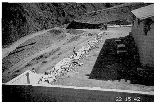
Photo 21. Collapse of the block wall enclosing the site of a storehouse for farm products 1-2 km north of Pakdeh (Site No. 2 in Fig. 7).
