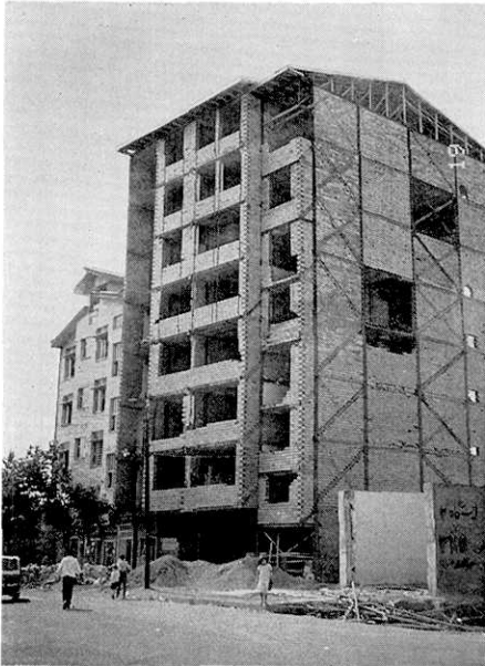
Photo 13. Tall building in Rasht. Eight-storied steel frame masonry structure. Some part of the bearing brick wall fell down. Wooden structure used under the roof.
