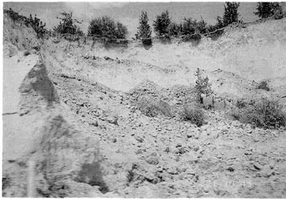
Photo 24. Slumping of a slope beside the road between Saravan and Rostam Abad (Site No. 2 in Fig. 6). Looking west.
