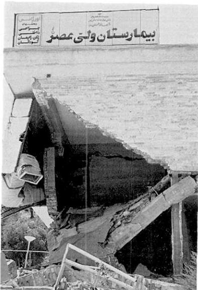
Photo 16. Same as Photo 15. The floor collapsed due to damage to the concrete columns and timbers.
