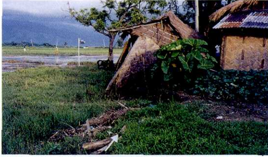
Photo 3. Faulting at Balacat Laron near Bongabon. Horizontal slip is 2 m. Western side was uplifted by 0.5 m. Note that a nipa house directly astride the fault was damaged, but neighboring houses were not.
