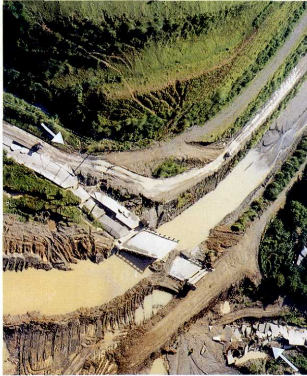
Photo 4. Aerial view toward the north showing collapsed concrete bridge north of Rizar. The fault runs just below the bridge spanning an irrigation canal. Many boulders were dislodged on the man-made terrace along the canal.
