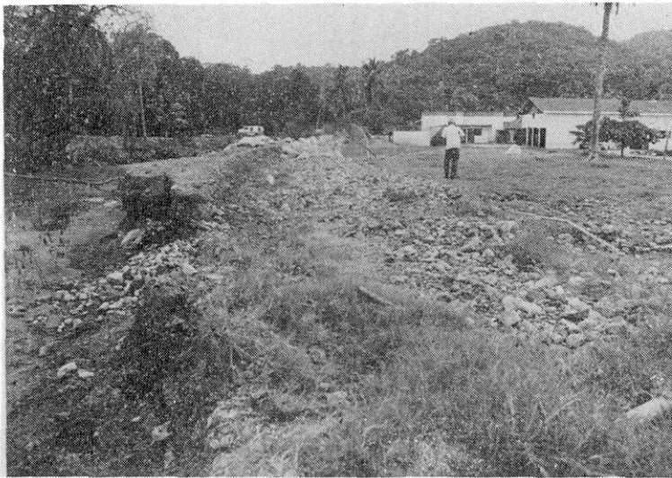
Fig. 5. Damage to the banks of the small stream at Playa Linda. The photo faces the sea.
