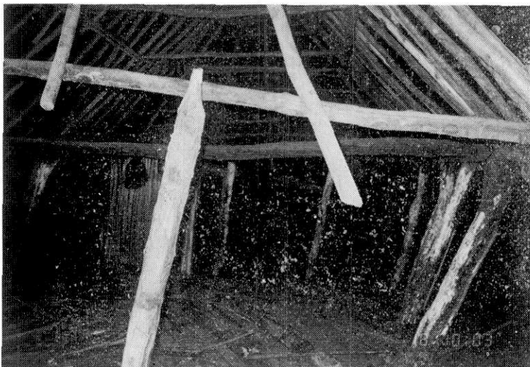
Fig. 3. Damage of thatched hut at Barra del Potosi. Pieces of furniture in the hut were washed away.
