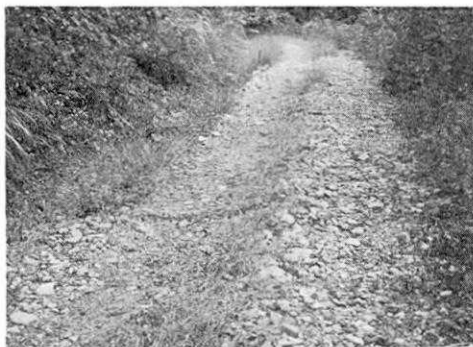
Fig. 33. En echelon cracks on a road at Loc. h (north of Satomiya), looking southeast.
