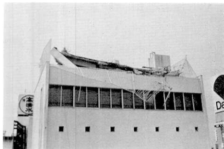
Fig. 13. Top part of the Honkin department store and its collapsed observatory. (Oh-machi, Akita city).
