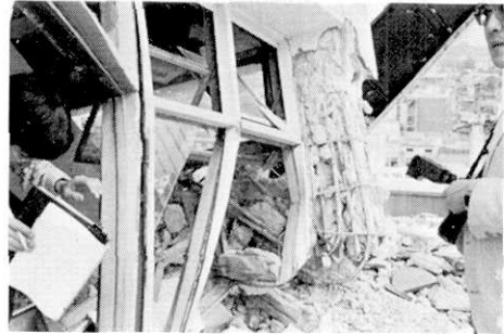
Fig. 15. Close up of damage to the column (Honkin Department Store, Akita city).
