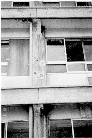
Fig. 4. Shear damage to column (Namioka town hospital).
