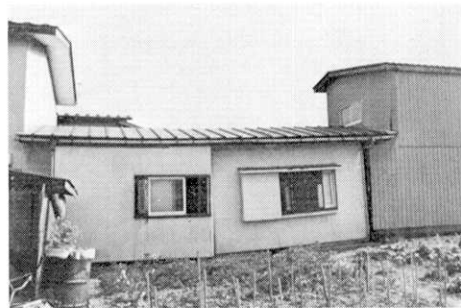
Fig. 5. Damaged wooden house due to subsidence of the ground (Arayamotomachi, Akita city).
