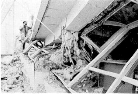
Fig. 14 Collapsed observatory (Honkin Department Store, Akita city).
