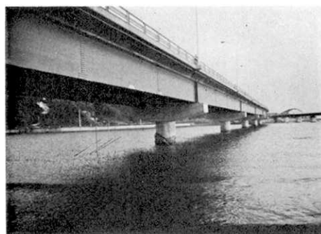
Fig. 43. Damaged No. 3 pier of Shizunai road bridge.
