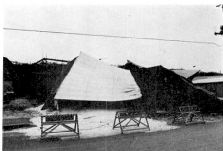
Fig. 15. Collapsed warehouse of a chip factory. (photographed by Urakawa town office.)
