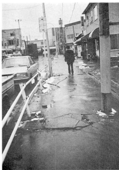
Fig. 8. Cracks in road pavement in Tokiwamachi in Urakawa town.
