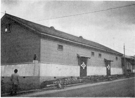
Fig. 37. Damaged warehouse made of mortar brick and mud in Mitsuishi town.
