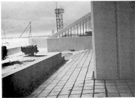
Fig. 19. Cracked pavement at entrance of Urakawa family sports center.
