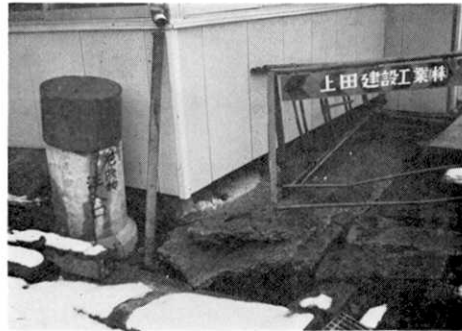
Fig. 10. Damaged foundation of the public bath.
