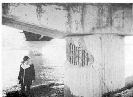
Fig. 41. Damaged No. 2 pier of Shizunai road bridge.
