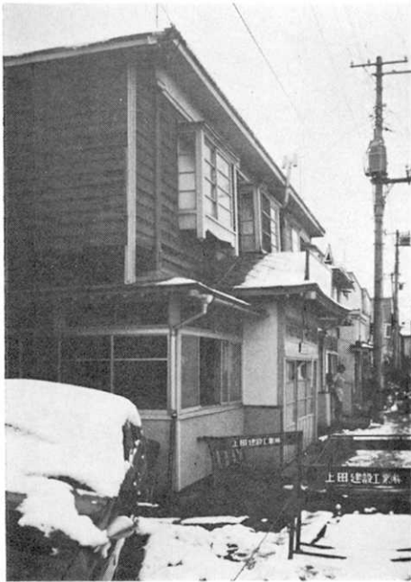
Fig. 9. Damage to a public bath in Tokiwamachi.
