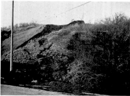
Fig. 52. Small scale landslide along national road No. 235.
