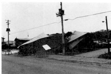
Fig. 14. Collapsed warehouse of a chip factory. (photographed by Urakawa town office.)
