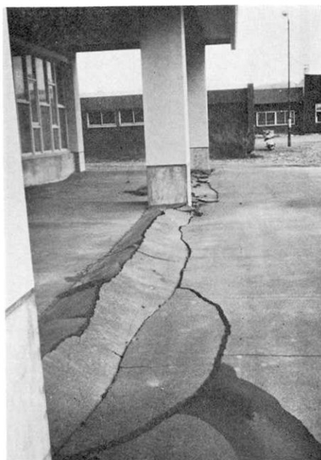
Fig. 36. Ground deformation at the entrance of Mitsubishi town sports center.
