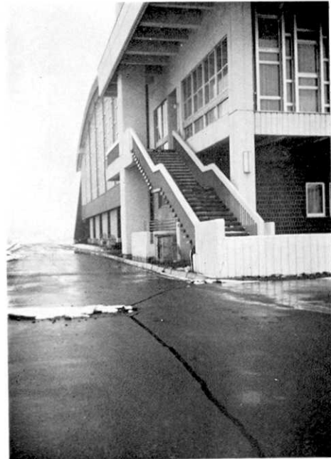
Fig. 20. Cracked pavement close to Urakawa family sports center.
