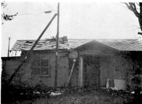
Fig. 32. Collapsed dwelling house of the schoolmaster of Mitsuishi primary school.
