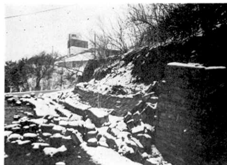
Fig. 46. Collapse of stone wall.
