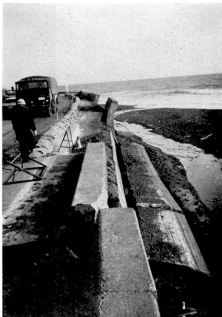
Fig. 47. Overturn of seawall.
