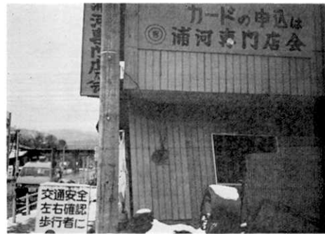
Fig. 11. Inclined house in Tokiwamachi.
