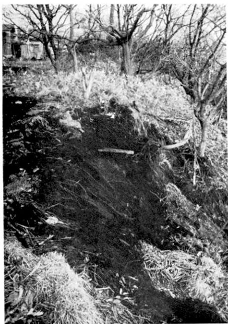
Fig. 34. Cliff slide just behind the schoolmaster's house.
