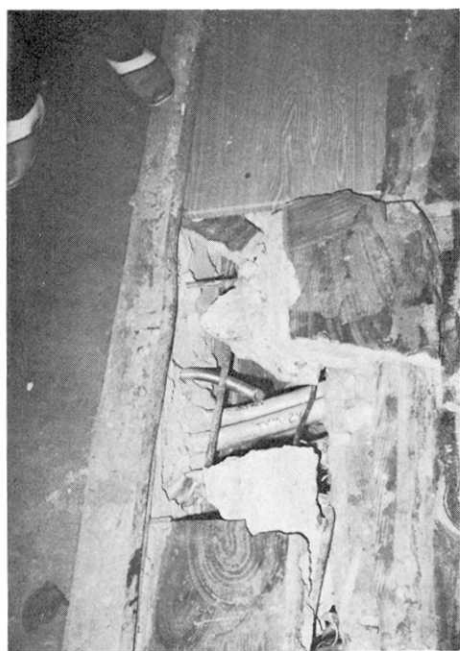
Fig. 16. Broken expansion joint in the reinforced concrete building of Urakawa primary school.
