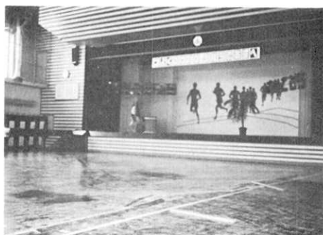
Fig. 17. Buckled floor of Urakawa primary school due to settlement of building resulting from collapse of pile foundation.
