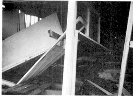
Fig. 31. Damaged toilet of Mitsuishi primary school.
