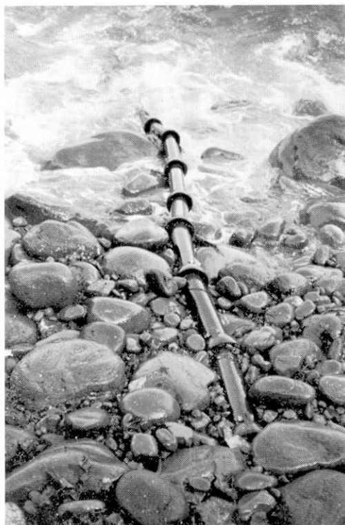
Fig. 11. The cable protected by an iron pipe on the seashore.
