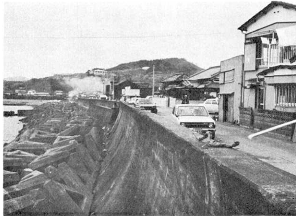
Fig. 3a. View of the sea wall at Kami-Kawaguchi. The 1854 Ansei tsunami ran into the town.
