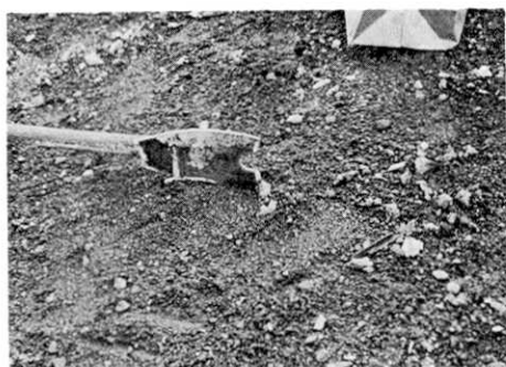
Fig. 11. Connector of brace broken at its profile deficiency (Futo Elementary School)
