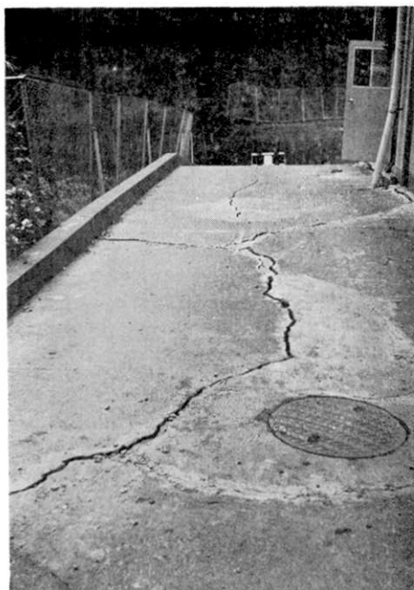
Fig. 3. Crack appeared on the west end of the lot (Futo Elementary School)
