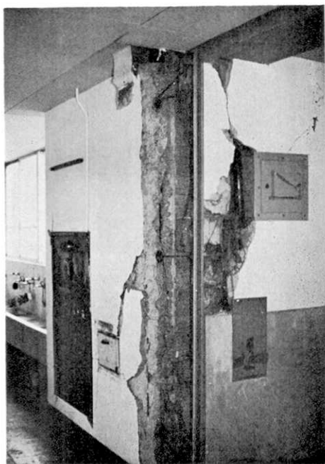
Fig. 5. Damage and crumbling of the facing (Futo Elementary School)
