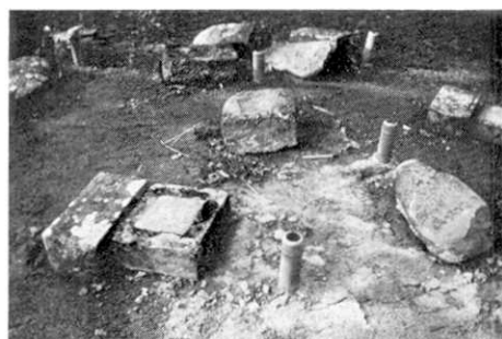
Fig. 21. Close up of Fig. 20. Crack in the ground shows softness of the ground.
