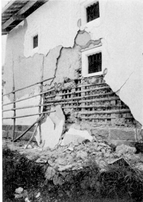
Fig. 25. This damaged warehouse is also located on a 2 m high embankment.
