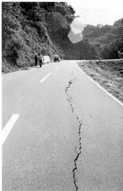
Fig. 7. Small crack in road pavement.
