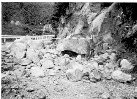
Fig. 10. A large amount of rock fell down on the road from a cut slope.
