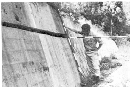
Fig. 12. Horizontal gap in the concrete retaining wall.
