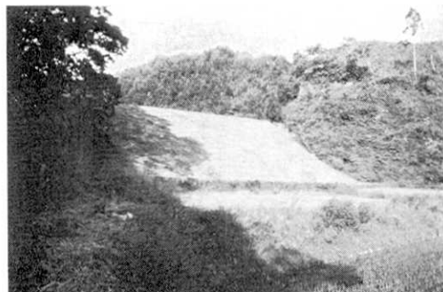
Fig. 18. An earthdam with an almost empty reservoir close to the damaged area suffered no damage.
