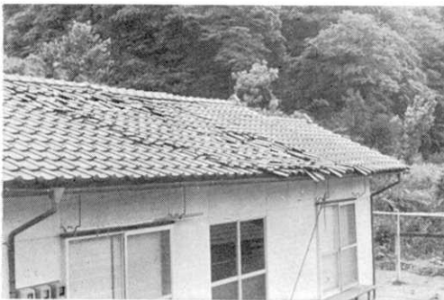
Fig. 6. Typical damage to a tile roof.
