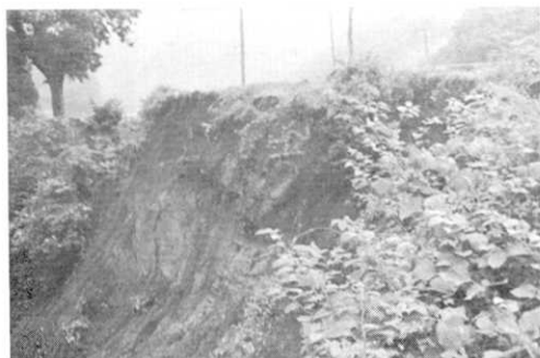
Fig. 13. Small scale landslide on a road embankment.
