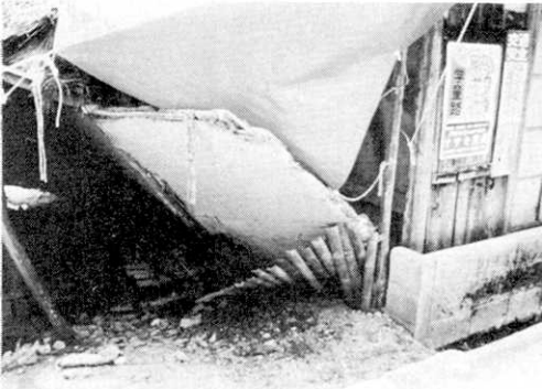
Fig. 2. Collapse of the clay wall of a straw thatched house.
