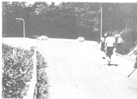
Fig. 9. Crack in the parking lot of the Sanbe hot spring appeared along a connecting part between an old road and a newly filled area.
