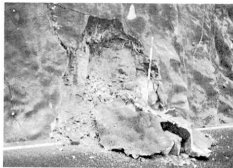
Fig. 11. Cement mortar for protection from small slides of the surface of the slope was also broken, a slide on a larger scale did not occur owing to the covered mortar.
