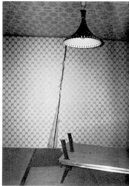
Fig. 5. A crack on a wall in a hotel room. The crack appeared on the joint with no reinforcement between the main building and the extended part.
