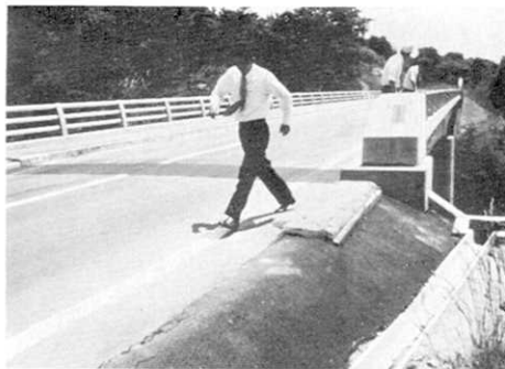
Fig. 8. Vertical gap between "Yunotani" bridge and an approaching embankment appeared after the earthquake and was repaired by pitch material.
