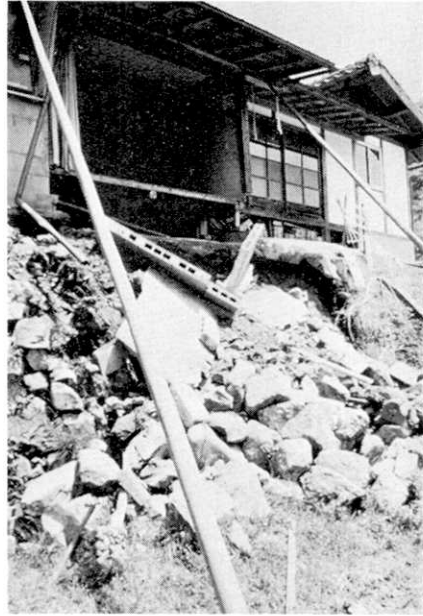
Fig. 3. Inclined floor of a wooden house due to fall of a stone wall.
