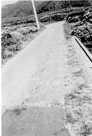
Fig. 10. Cracks in a concrete pavement.
