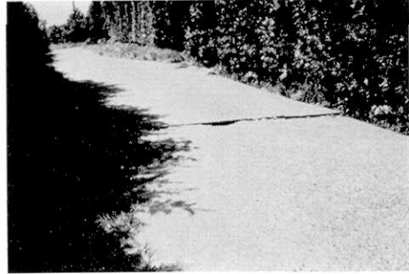
Fig. 9. Vertical offset appeared in a concrete pavement.
