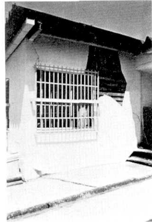
Fig. 7. Damage to a wall.
