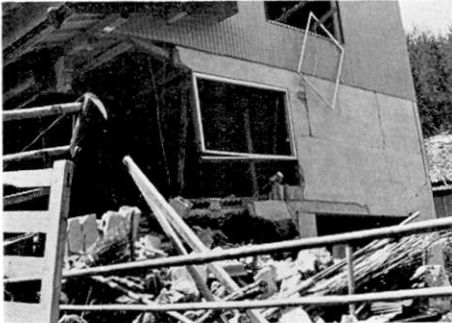
Fig. 38. Damage to a warehouse at Ogiyama.
