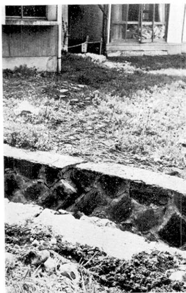
Fig. 21. Fissures in the ground by the boarding house for employees of hotel at the side of Yamashita-ike.
