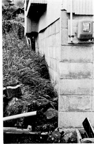
Fig. 40. Distortion of a warehouse by a left-lateral displacement along the fissures in the ground at Ogiyama.
