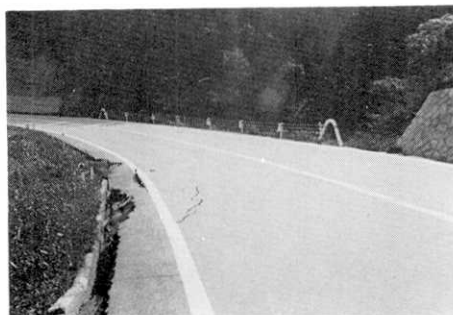
Fig. 67. Damage to Yamanami Highway at 8.5 km curve, where fault ② crosses. No indication of surface faulting.
