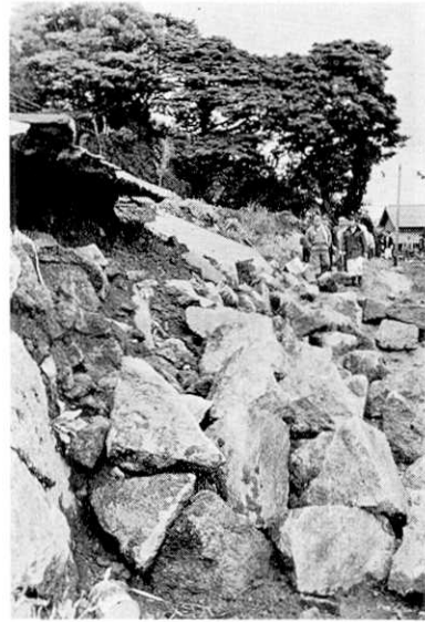
Fig. 45. Sliding of supporting soil of a house garden at Uchiyama.
