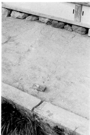
Fig. 75. Ground cracks and left-lateral offset of concrete blocks (Mr. Kai's house).
