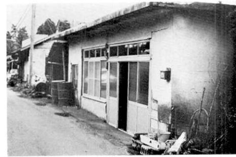
Fig. 60 b Damage at Senchomuda failure of the wall of a house made of concrete-block (already sepaired).
