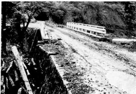
Fig. 39. Damage to a bridge at Ogiyama.
