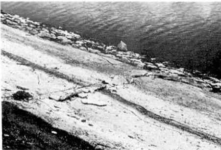
Fig. 24. Cracks on a concrete-wall of an earth-dam (Yamashita-ike Dam).
