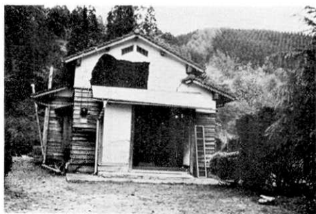
Fig. 14. Damage of a house of the Kyushu-Rinsan Inc. at Teradoko.
