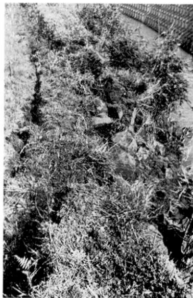
Fig. 56. Sliding of supporting wall by a river at Shimodakita.
