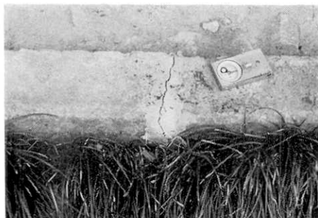
Fig. 76. Cracks after repairing, showing after-slip movements (location same as Fig. 75).
