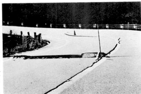
Fig. 29. Cracks on the Yamanami Highway at point No. 477 (9.5 km) on the trace of an active fault, near Yamashita-ike.
