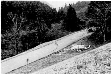
Fig. 23. Cracks on an asphalt-road at the side of Yamashita-ike.
