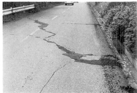
Fig. 63. Cracks on a paved road on the fault line ①, ca. 30 meters north of a fork to the Lakeside Hotel, looking northwest. Photo was taken after repairing.
