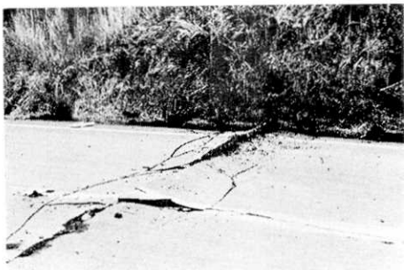
Fig. 27. Pressure-ridge-like cracks on the Yamanami Highway near Yamashita-ike at point No. 523 (10.4 km).
