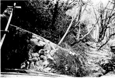
Fig. 22. Fissures in the ground and destruction of stone wall (already repaired) by a rest-house at the side of Yamashita-ike.
