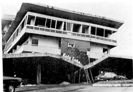
Fig. 17. Damage of a hotel (Lakeside Hotel) at the side of Yamashita-ike.
