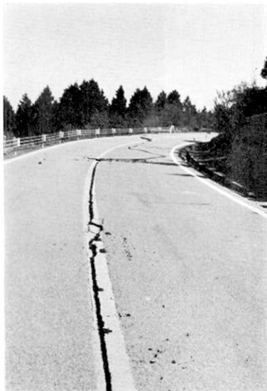
Fig. 30. Cracks on the Yamanami Highway at point No. 457, (9.1 km near Yamashita-ike).
