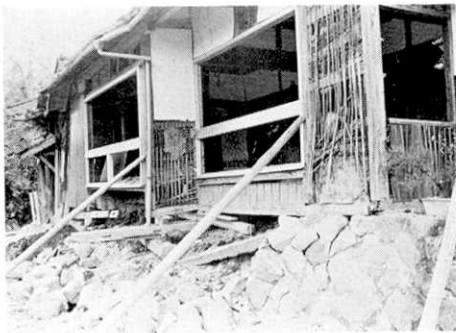
Fig. 48. Damage to a house at Ageju. (Mr. Hitoshi Ito's house).
