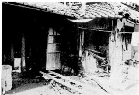
Fig. 52. Damage to a house at Shiode.
