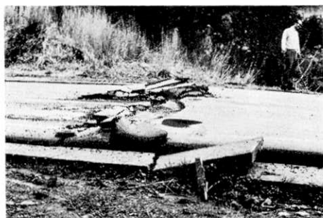
Fig. 28. Pressure-ridge-like cracks on the Yamanami Highway near Yamashita-ike at point No. 481 (9.6 km).
