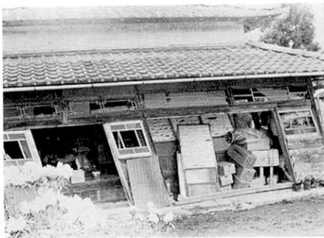
Fig. 49. Damage to a house at Ageju. (Mr. Yoshinobu Ito's house).
