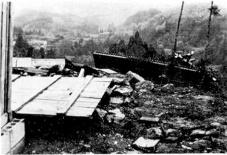
Fig. 7. Collapse of a shrine at Okunameshi.
