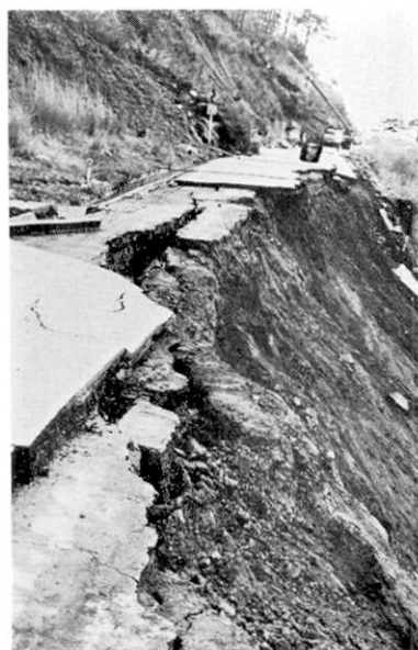
Fig. 31. Collapse of the Yamanami Highway at point Nos. 416~422 (8.3 km), at Yamashita-ike.
