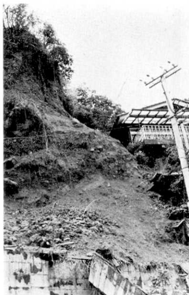
Fig. 35. Sliding on a cliff wall at Yunohira.
