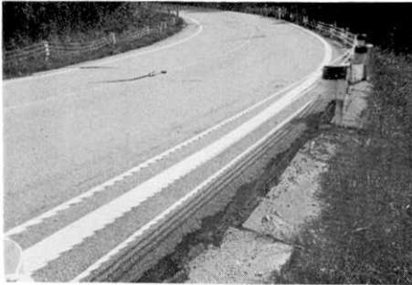
Fig. 69. Damage to Yamanami Highway at 9.5 km curve, where fault ③ crosses. No indication of surface faulting.
