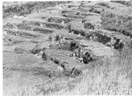
Fig. 59 b. Damag at Hata, slidin of supo rting stone walls of rice fields.
