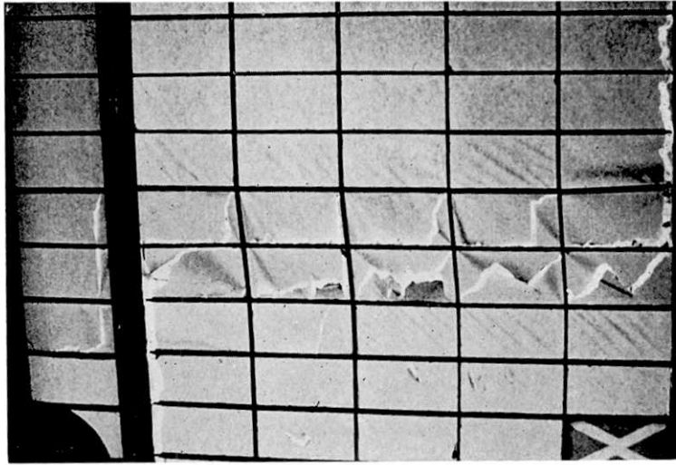
Fig. 4. Break of the shoji in a house. Figure shows clearly that it was broken due to a shearing stress. (Hatasa section, Okumyogata Village)
