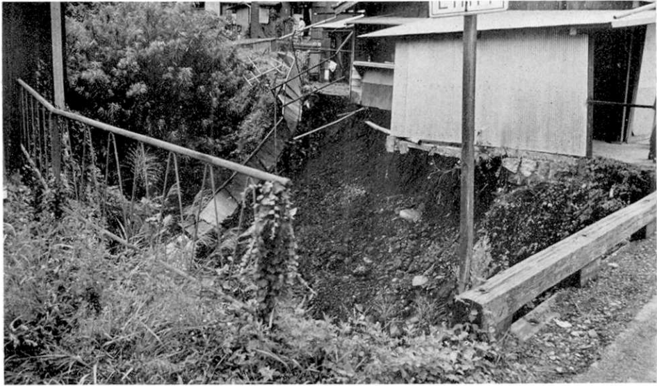
Fig. 2. Example of a failure of the fill-up foundation of a house. (Gujoyochachiman Town)
