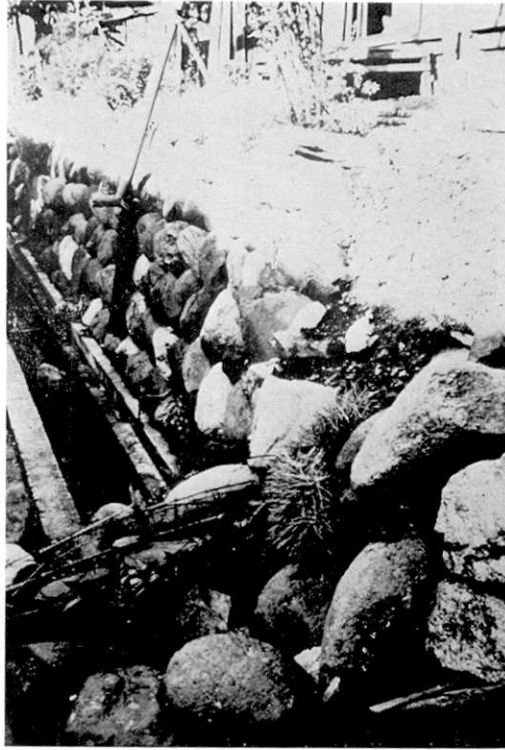
Fig. 6. Failure of the masonry retaining wall. (Okumyogata Village)
