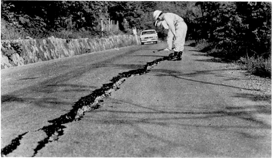
Fig. 8. Occurrence of a crack in the pavement due to the slide of the roadbed. (Prefectural road, from Hachiman to Kanayama, Horigoshi mountain pass)
