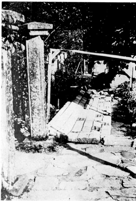
Fig. 12. Example of a collapse of the block-wall. (Gujoyohachiman)
