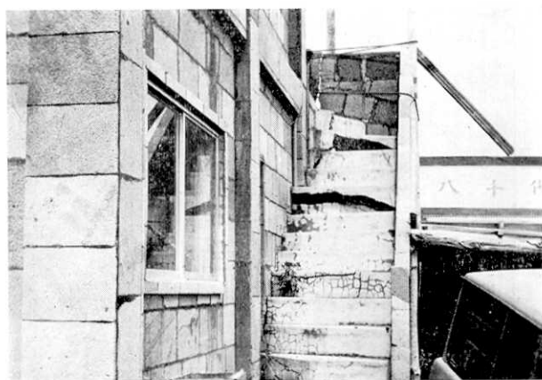
Fig. 17. Damage to house at Sikine-zima.
