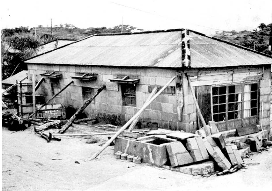
Fig. 19. Damage to house at Sikine-zima.
