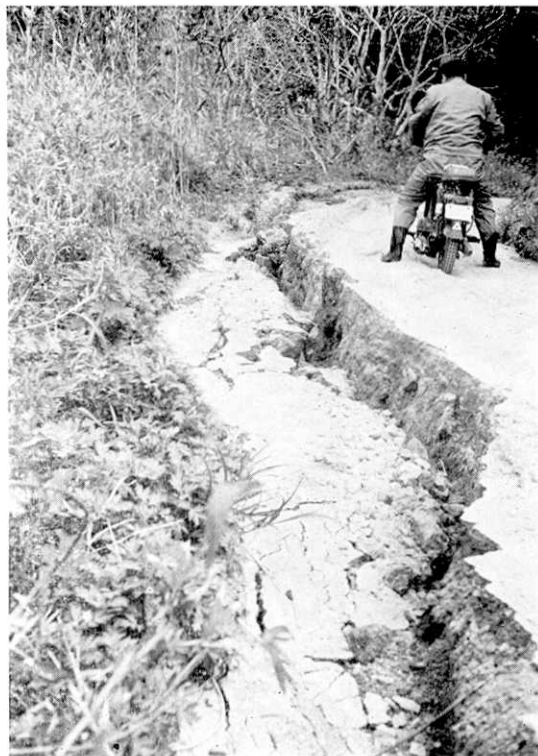
Fig. 13. Cracks made on the road of Kozu-sima.
