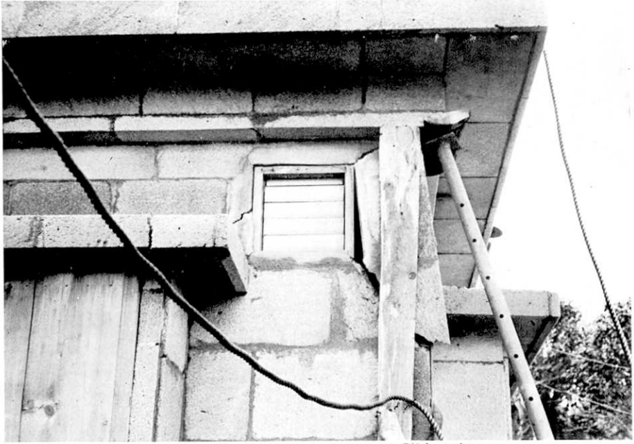
Fig. 18. Damage to house at Sikine-zima.
