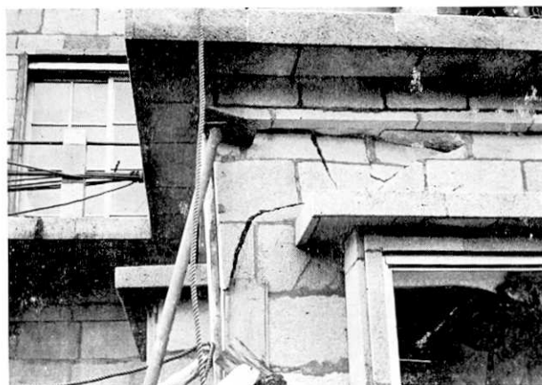
Fig. 16. Damage to house constructed of "Koga-seki", vesicular rhyolite lava, at Sikine-zima.
