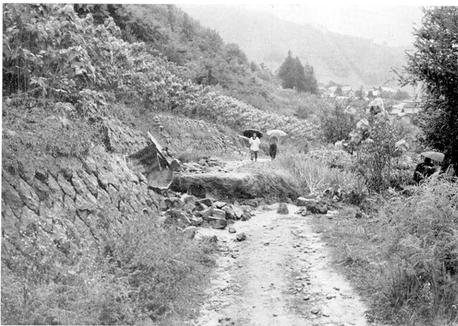
Fig. 4. A rural road was cut through by one of the cracks along which the anticipated landslide was going to occur. Displaced height was about 80 cm, 20 minutes before the visible sliding started. Horizontal lines were marked for levelling on the stone wall at the left side of the road.
