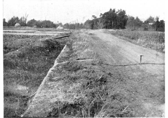
Fig. 2. Earthquake rift nr. Simo
