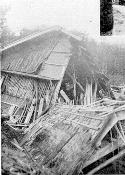
Fig. 39 A house at the village of Go (郷), under which a fault scarp was formed.
