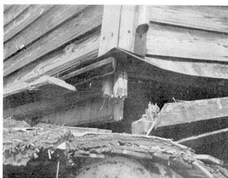
Fig. 17 A post fractured at the connection to the second story beam.
