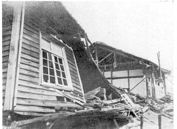
Fig. 15 Broken at the first and second stories.
