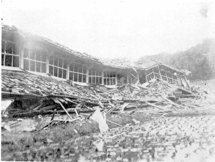
Fig. 9 An example of bad construction, roofed with heavy tiles and having no braces.
