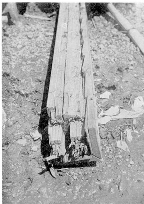
Fig. 18 The fracture of a post.
