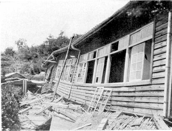
Fig. 14 Broken at the first story.
