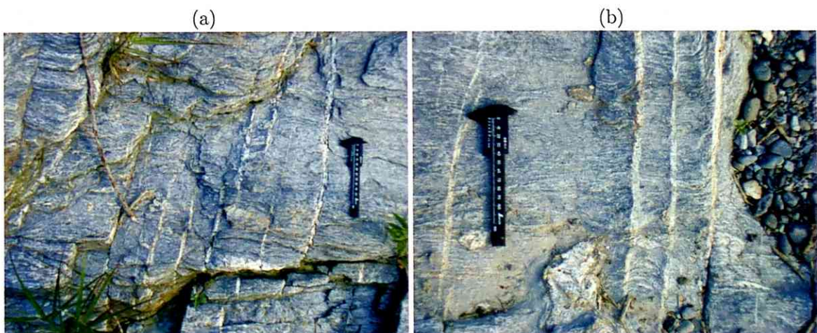
Figure.3-4 Sealed cracks cutting schistosity planes with high angle. Observed (a)obliquely upward on the schistosity planes (b)just above the schistosity planes. Location:Shiratori bridge.
