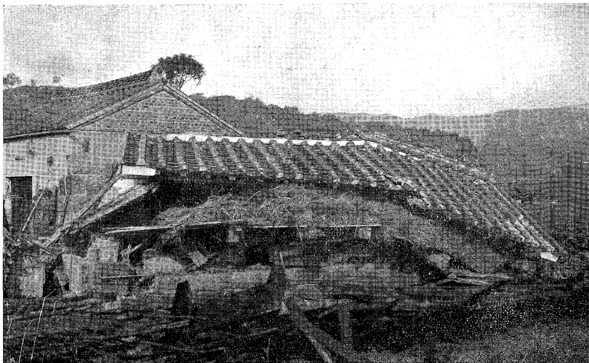
A warehouse at Hashiguchi, Kita-Arima. Its longer side was parallel to NNE.
