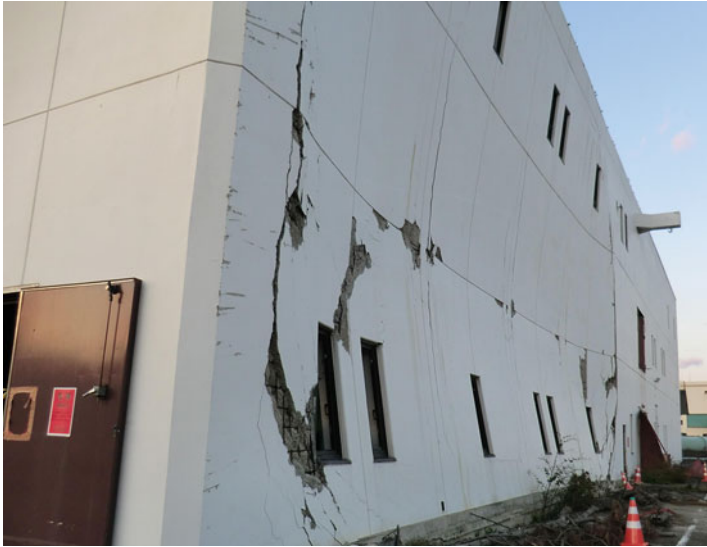
Fig. 2.9 Wall at wastewater treatment plant collapsed by tsunami
