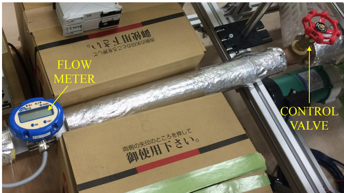
Figure 6-4: Flow meter installation downstream from the control valve.
