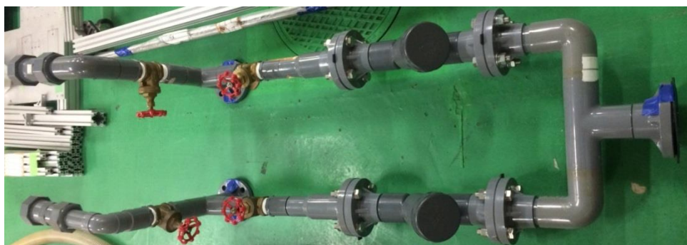
Figure 5-5: A portion of PVC piping in the loop.
