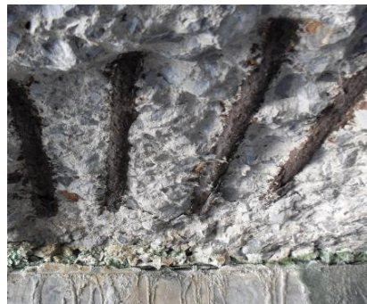
Figure 1-1 Corrosion and spalling of reinforced concrete (RC) structure in Rayong province, Thailand caused by airborne chloride.
