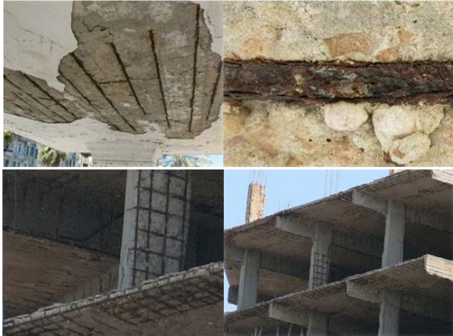
Figure 2-2 Existing RC residential structures suffering from heavy corrosion caused by airborne chloride attacks from the Mediterranean Sea in Alexandria, Egypt (2013) [7].
