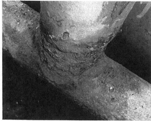
Figure 1.1. CUI located at tee pipe discontinuity [17]
