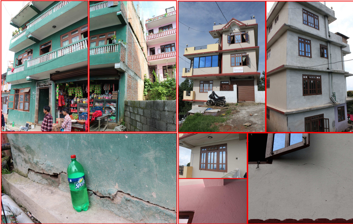
(a) Building 9 and its corresponding damaged state in the field study conducted in Nepal (b) Building 11 and its corresponding damaged state in the field study conducted in Nepal
