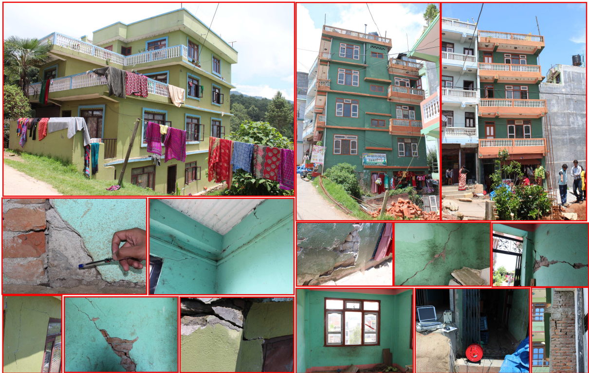
(a) Building 12 and its corresponding damaged state in the field study conducted in Nepal
