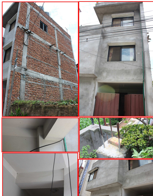
(b) Building 13 and its corresponding damaged state in the field study conducted in Nepal
